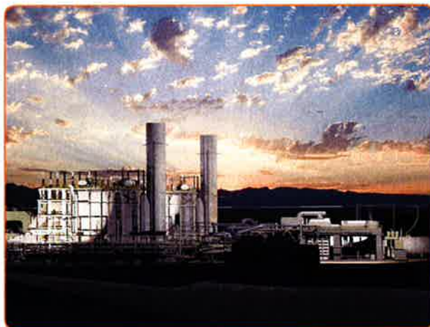
Harry Allen Generating Station, Las Vegas, Nevada
