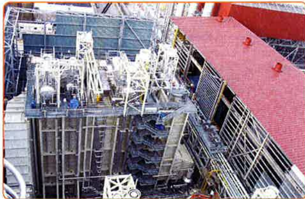
Astoria Power Plant, New York City, New York
