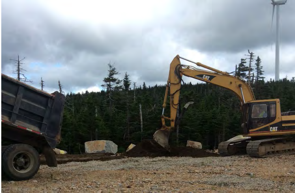
Figure 1: Pad 10: soil spread with excavator (to decrease soil compaction), Dump truck placing soil on pad area delineated with paint. Excavator operator is spreading to specified soil depth for specific pad depths. Machine was then used to tread site once for soil stabilization.
