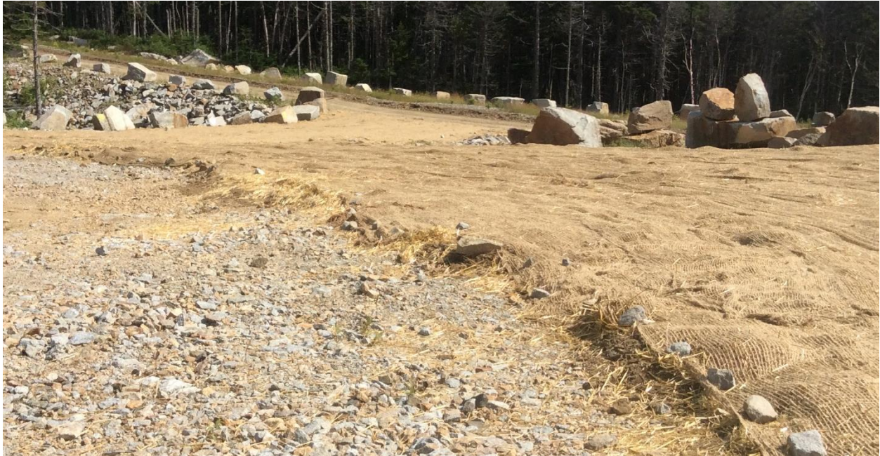
Figure 6: Pad 13- Ready for planting with 4 inches of soil, straw and Jute erosion cloth
