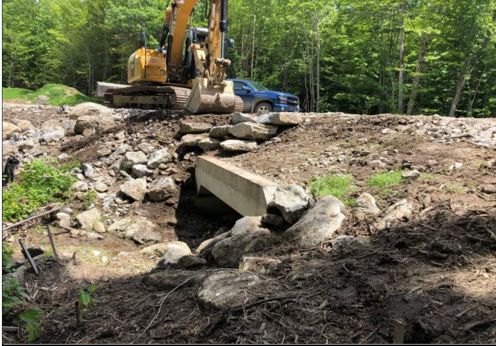
Photo No. 3 Photo Date: June 27, 2019 Site Location: Box Culvert Outlet, Antrim Wind Park, NH Description: Placed large boulders to stabilize slope and roadway and pulled top of slope back above headwall and compacted gravel and smaller rip rap. Photo By: JMM
