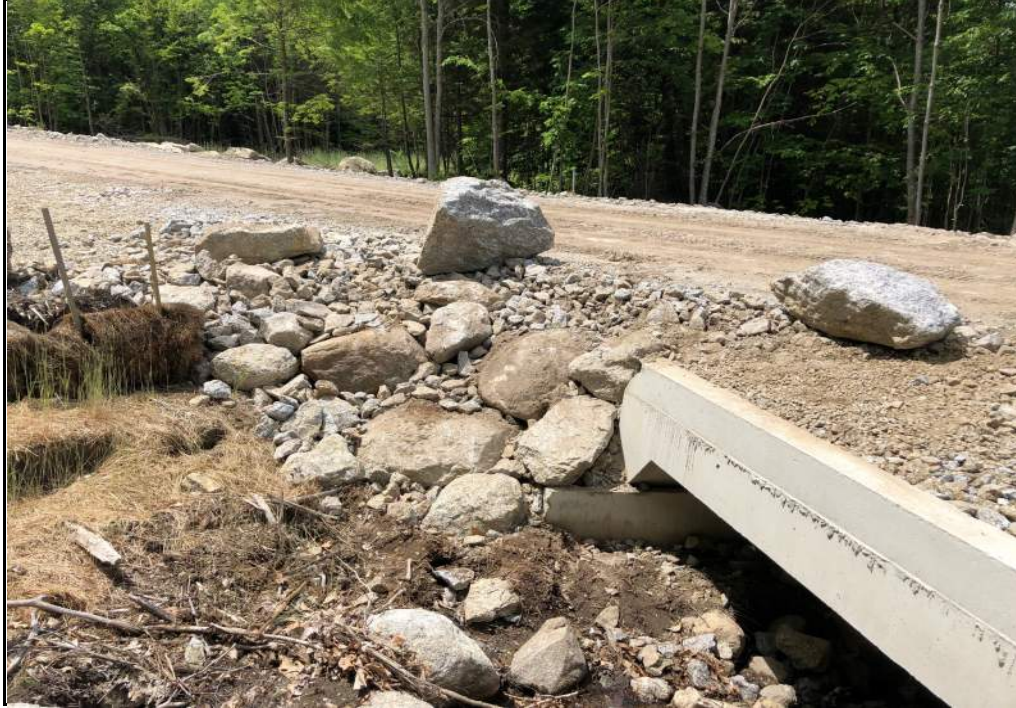
Photo No. 1 Photo Date: June 27, 2019 Site Location: Box Culvert Inlet, Antrim Wind Park, NH Description: Cleaned up loose gravel and compacted along headwall/deck of box culvert. Photo By: JMM
