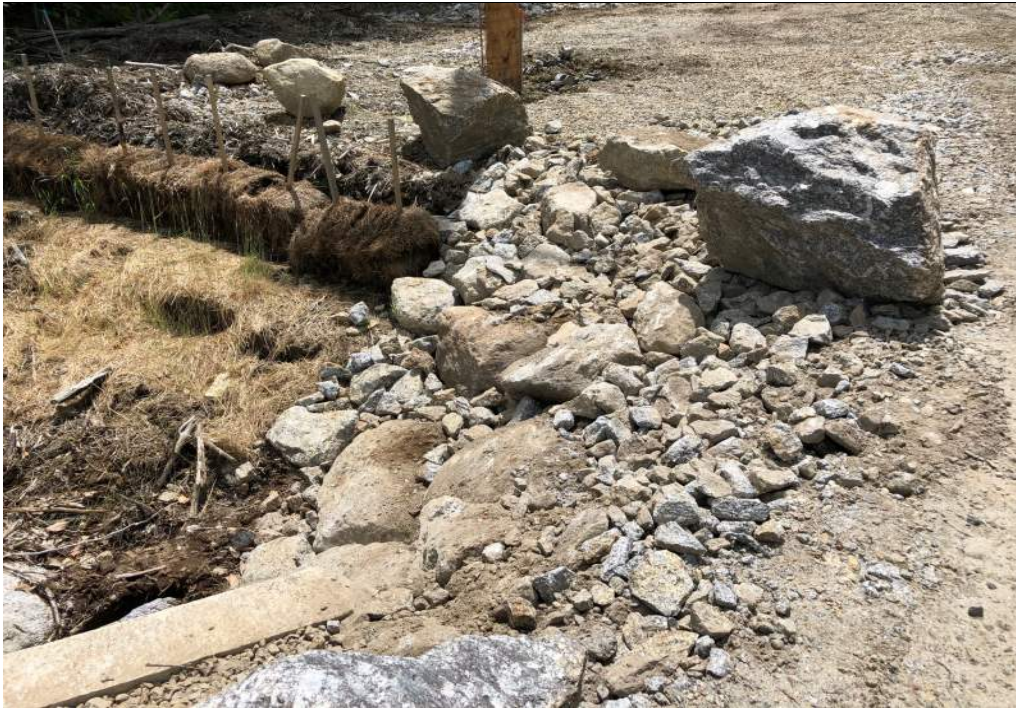
Photo No. 2 Photo Date: June 27, 2019 Site Location: Box Culvert Inlet, Antrim Wind Park, NH Description: Pulled back top of slope and filled in voids around boulders with smaller rip rap to avoid any erosion. Photo By: JMM
