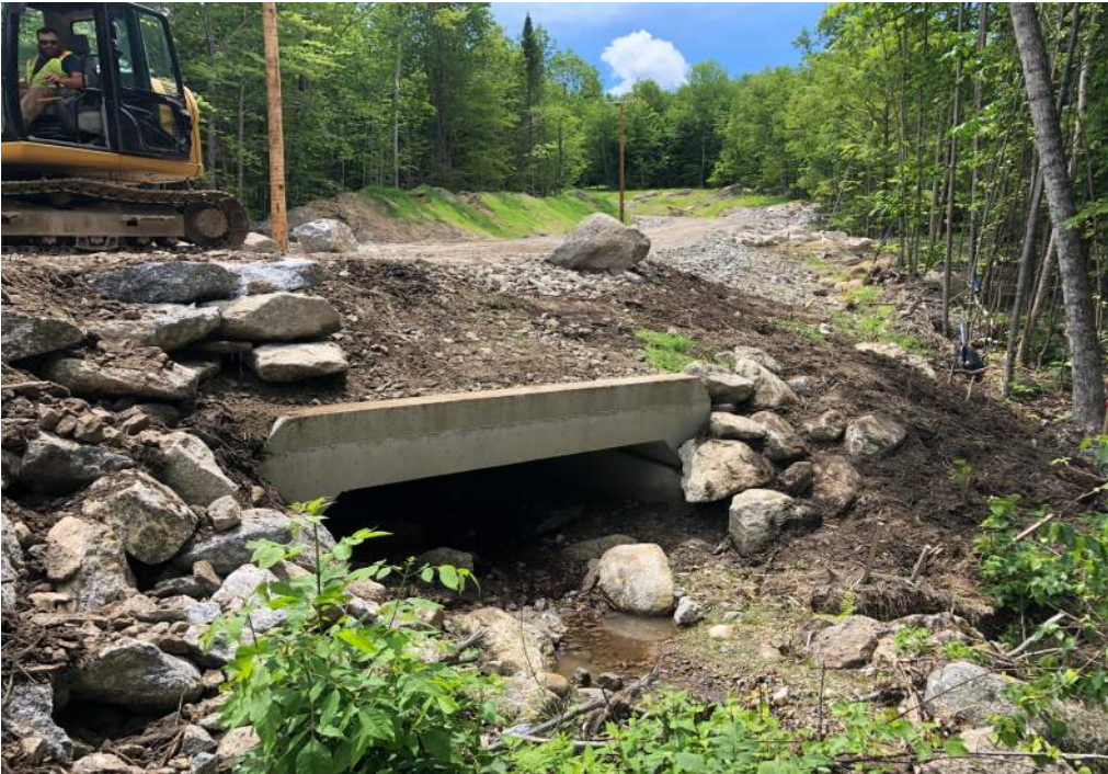
Photo No. 4 Photo Date: June 27, 2019 Site Location: Box Culvert Outlet, Antrim Wind Park, NH Description: Cleaned up stump grindings and lose material above headwall and slope around boulders that had potential of falling into stream Photo By: JMM
