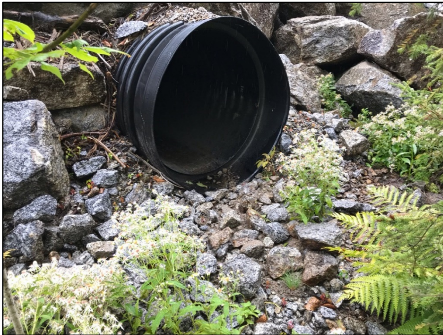
Photo 4: Image taken on 9/12/2019. Image showing fill and small diameter blast rock has been added to raise the elevation of the ground upstream of the inlet at culvert SD-26, alleviating the perched condition of the culvert inlet. Corrective actions to address perched conditions were taken prior to receipt of the letter from NHDES dated 9/10/2019.
