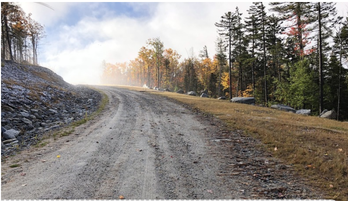
View of crane path and vegetated area adjacent to crane path at STA 135+00.
