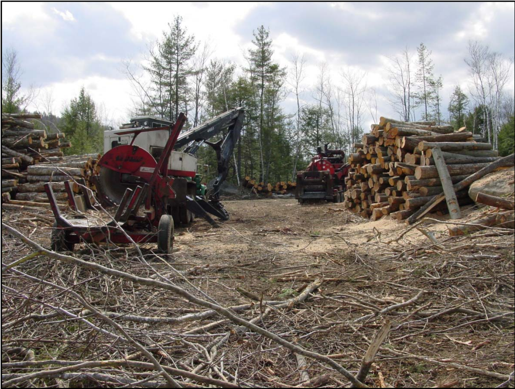
Figure 2. Log landing with slasher (left), chipper (right), and wood sorted by product.
