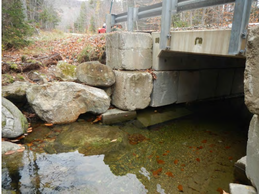
Photo 3. Pre- Emergency Authorization - Looking north at the southwest corner of abutment #1 (upstream side)
