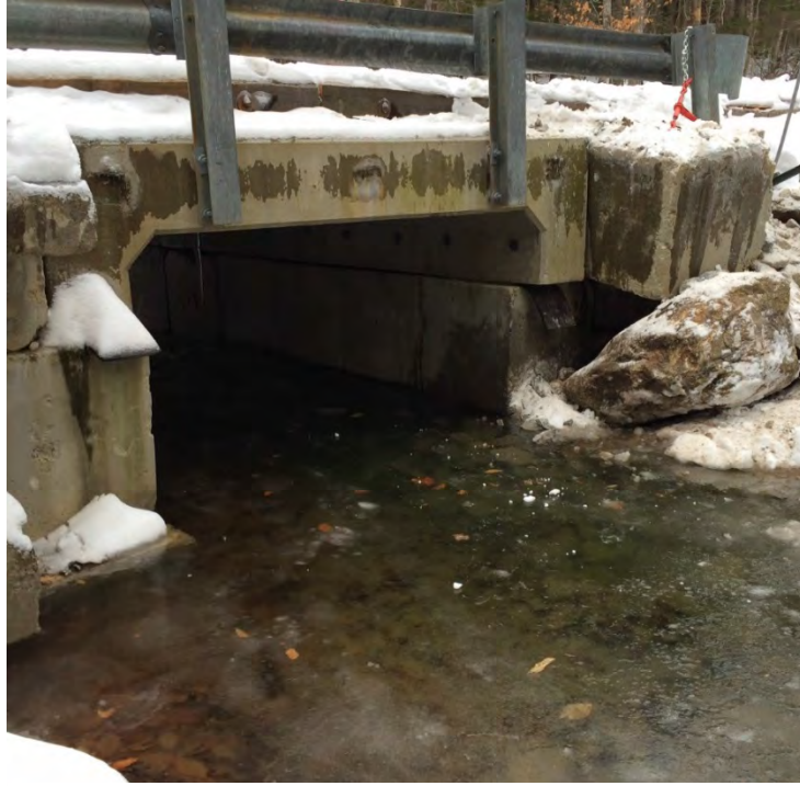
Photo 9. Post- Emergency Authorization - Looking west at Northwest corner of abutment #1 (downstream side).
