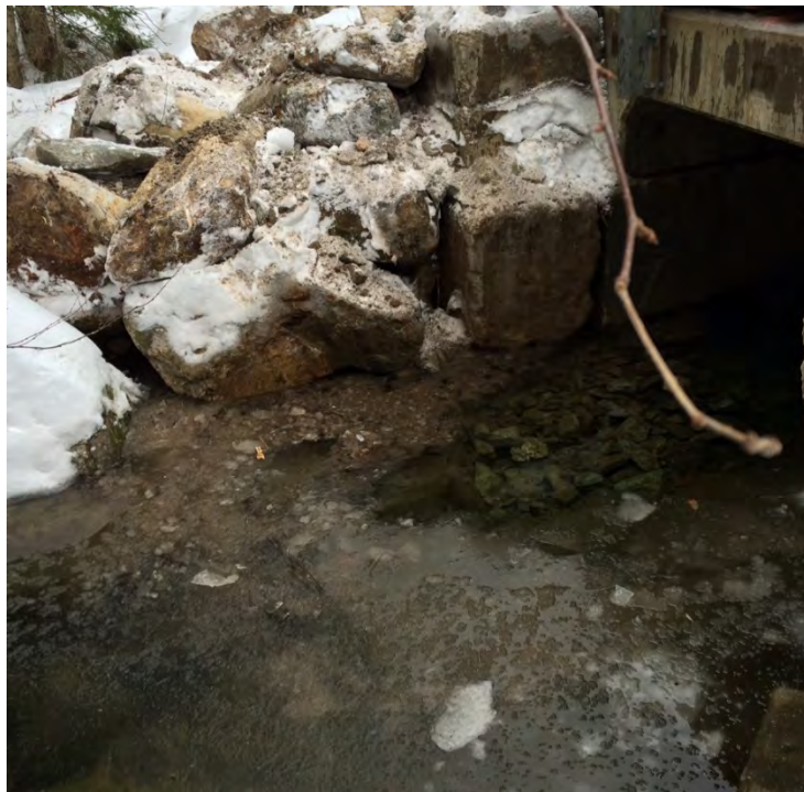
Photo 10. Post- Emergency Authorization - Looking north at the southwest corner of abutment #1 (upstream side)
