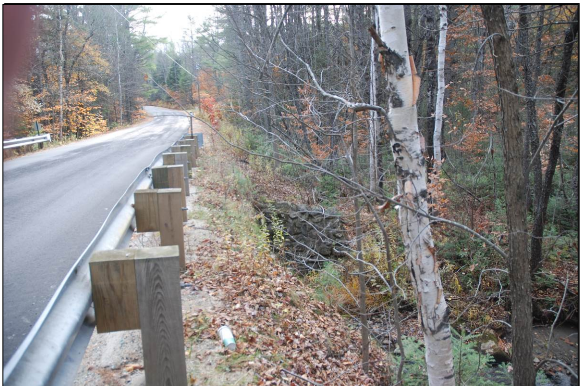
Photo 88 description: Wild Meadow Road, culvert over Hoyt Brook, VHB-GRA-010 (GRA0013), Grafton Roll: _____ Frame: _____ Direction: N Date taken: 12-2012 Negative stored: _____
