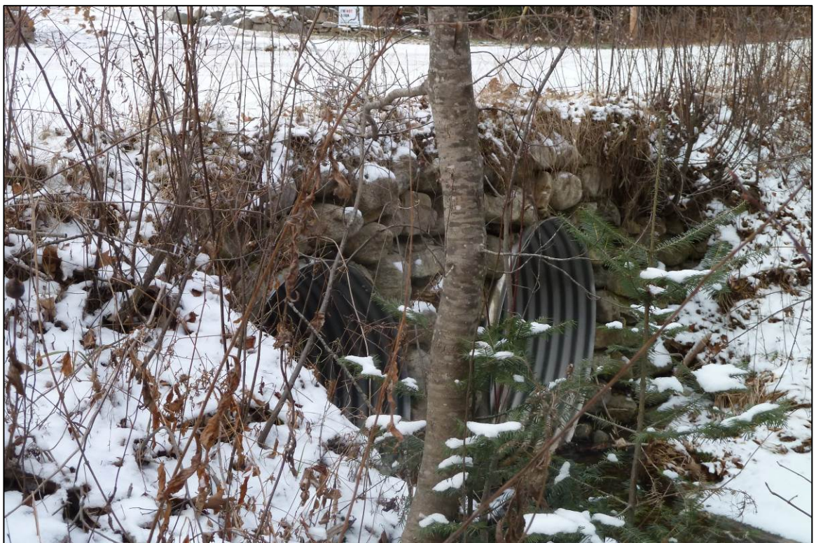
Photo 120 description: Gifford Hill Road over Hoyt Brook, VHB-GRA-013, Grafton Roll: _____ Frame: _____ Direction: N Date taken: 12-2012 Negative stored: _____
