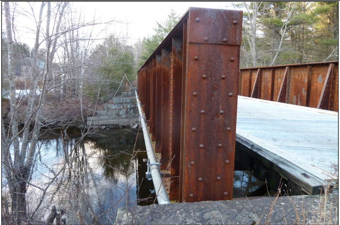
Photo 107 description: Former railroad bridge over Smith River, Ford Mill Road, VHB-DNB-008, Danbury Roll: _____ Frame: _____ Direction: N Date taken: 11-2012 Negative stored: _____
