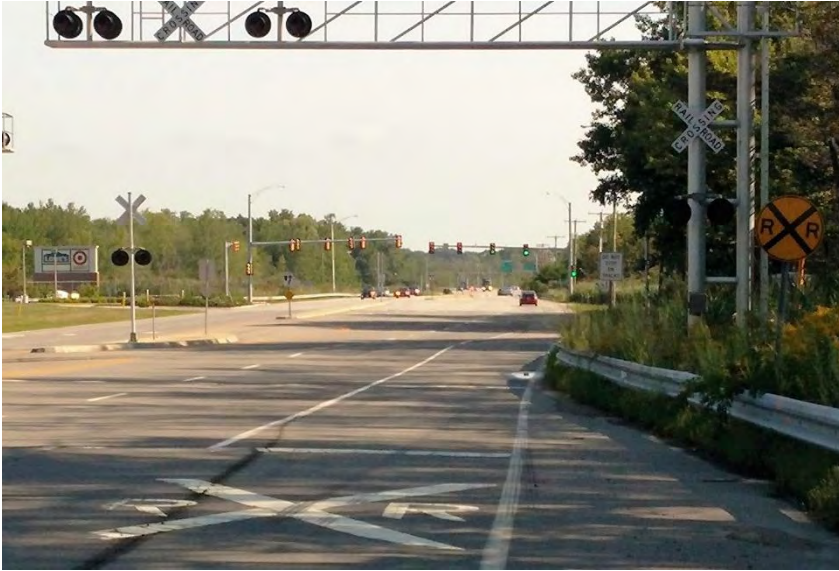
Greenland Rd - USDOT 054416P (no gates)
