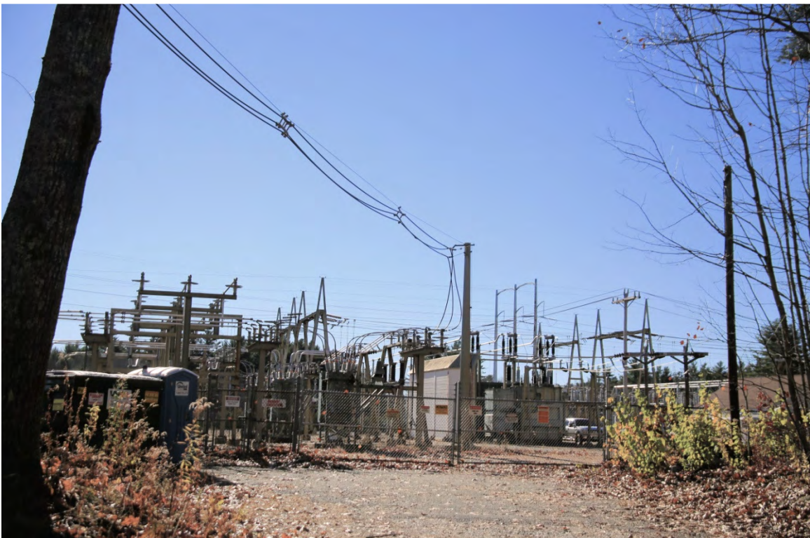
Photo 010) Miles Road – Madbury Substation Photo taken November 2015
