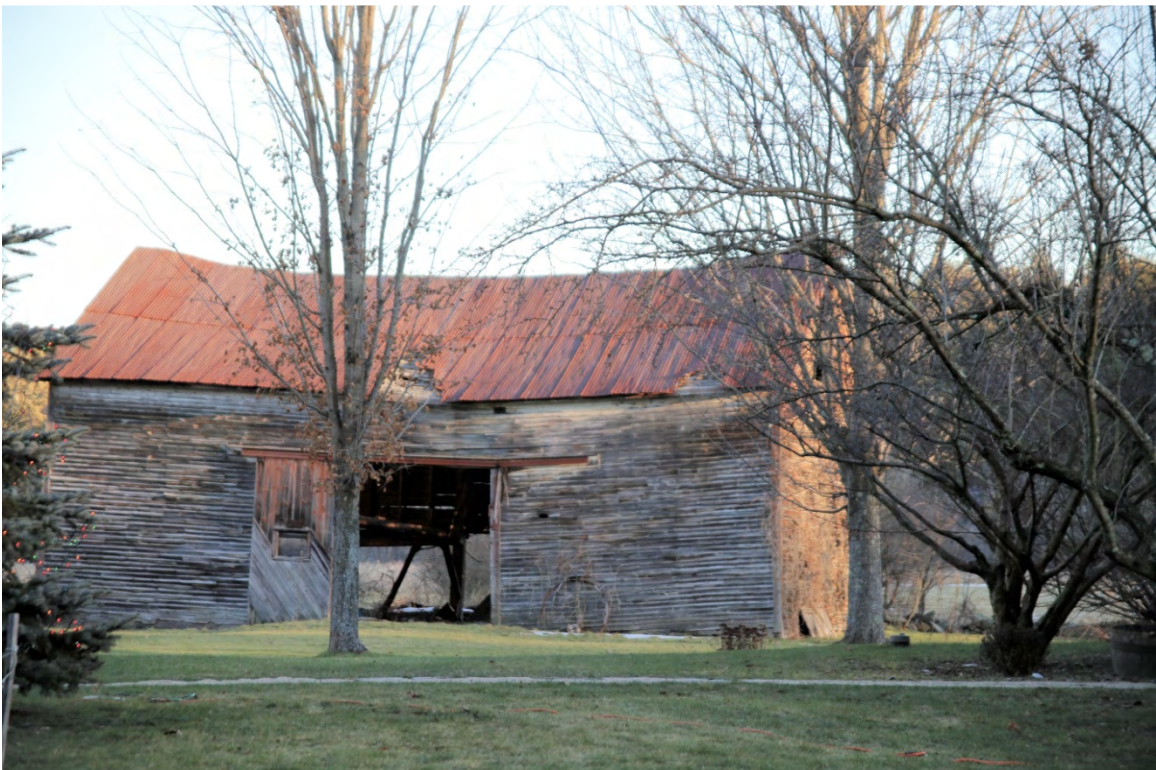
Photo 169) Newmarket-Bennett Road Farms Historic District – 97 Newmarket Road – Thompson-Pierre Hamel Farm (DUR0011) Direction: SE
