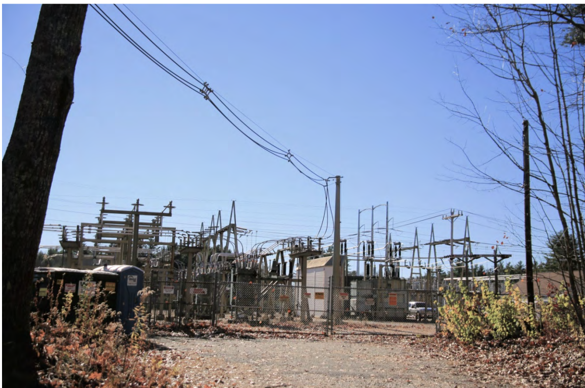
Photo 010) Miles Road – Madbury Substation Photo taken November 2015
