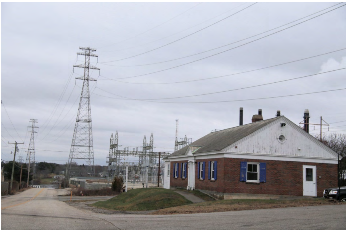
Photo 288) 300 Gosling Road (Portsmouth) – Schiller Power Plant office ID: N-87, photo taken December 2015
