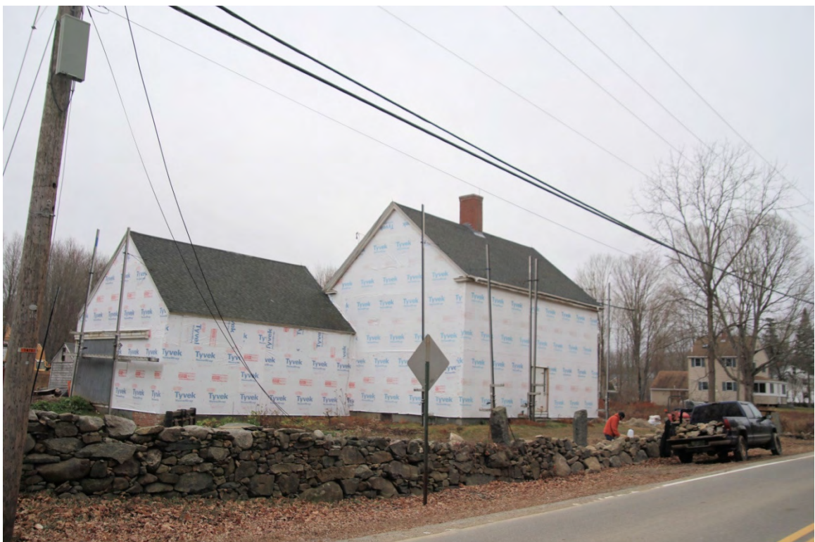
Photo 250) 233 Nimble Hill Road – Coleman House being remodeled (#129) ID: N-40, photo taken December 2015
