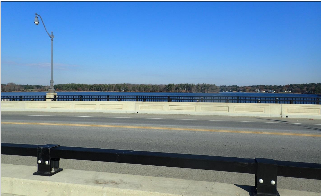
12. Views from Scammell Bridge from Route 4 (#75): View looking north over the bridge toward Clements Point
