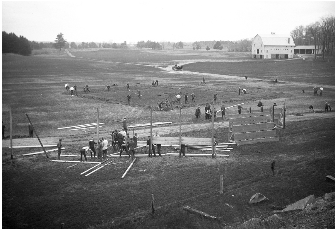
Brackett Field baseball field construction and horse barn (now vicinity of Cowell Stadium), 1921 (University of New Hampshire Library Digital Collections)
