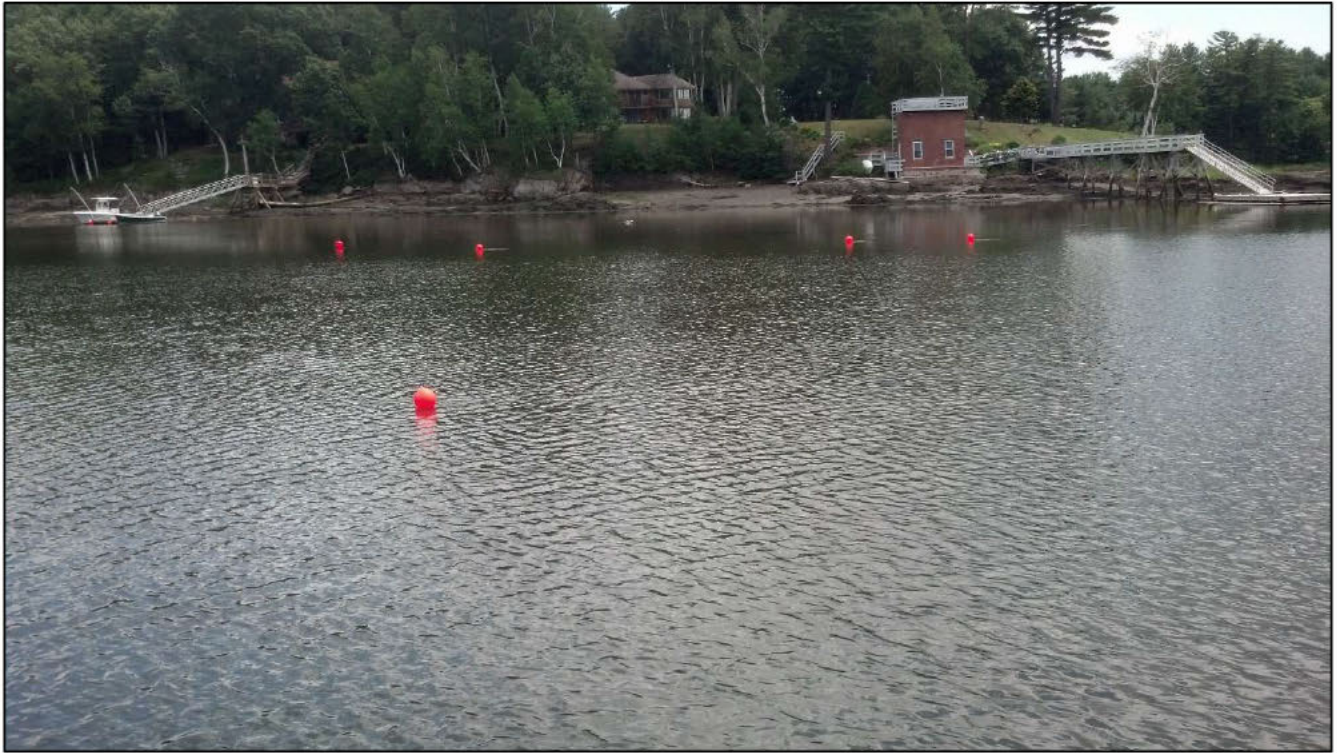
Figure 4: View of the work area at the Eastern Shore landing approach; floats were affixed to the as-found cables by divers.
