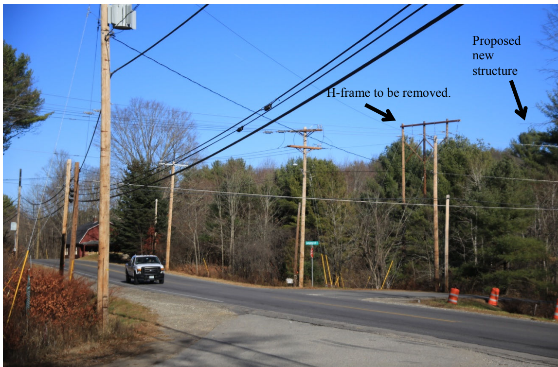
Electric utilities at Newmarket Road near the Bennett Road intersection, facing northwest. H-frame to be removed, all other structures and lines to remain in place
