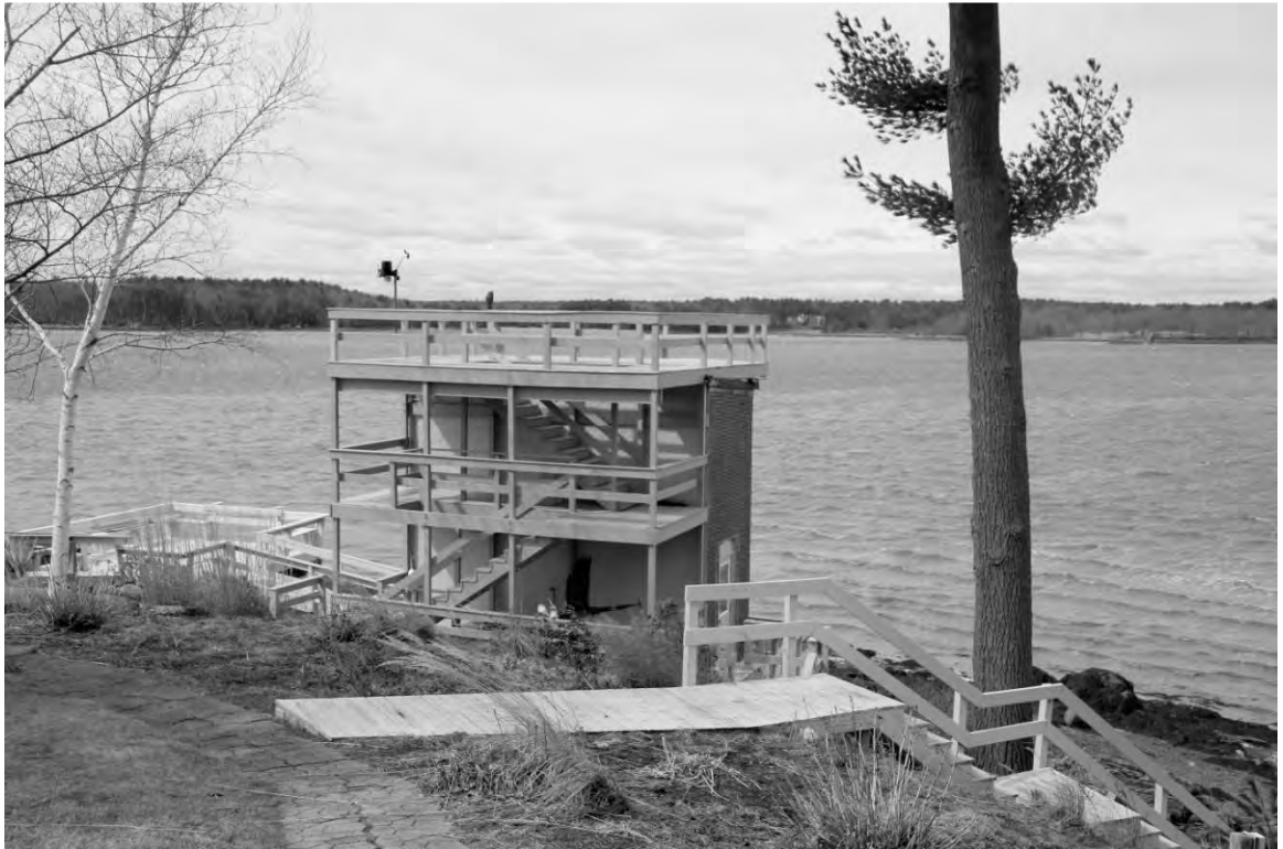
Photo 3) New stairs and deck on cable house from grounds of 44 Gundalow Landing Direction: SW
