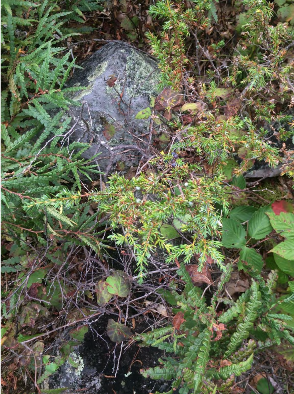
Dislodged rocks near breach in southern stone wall exhibiting growth of woody vegetation over the stone.
