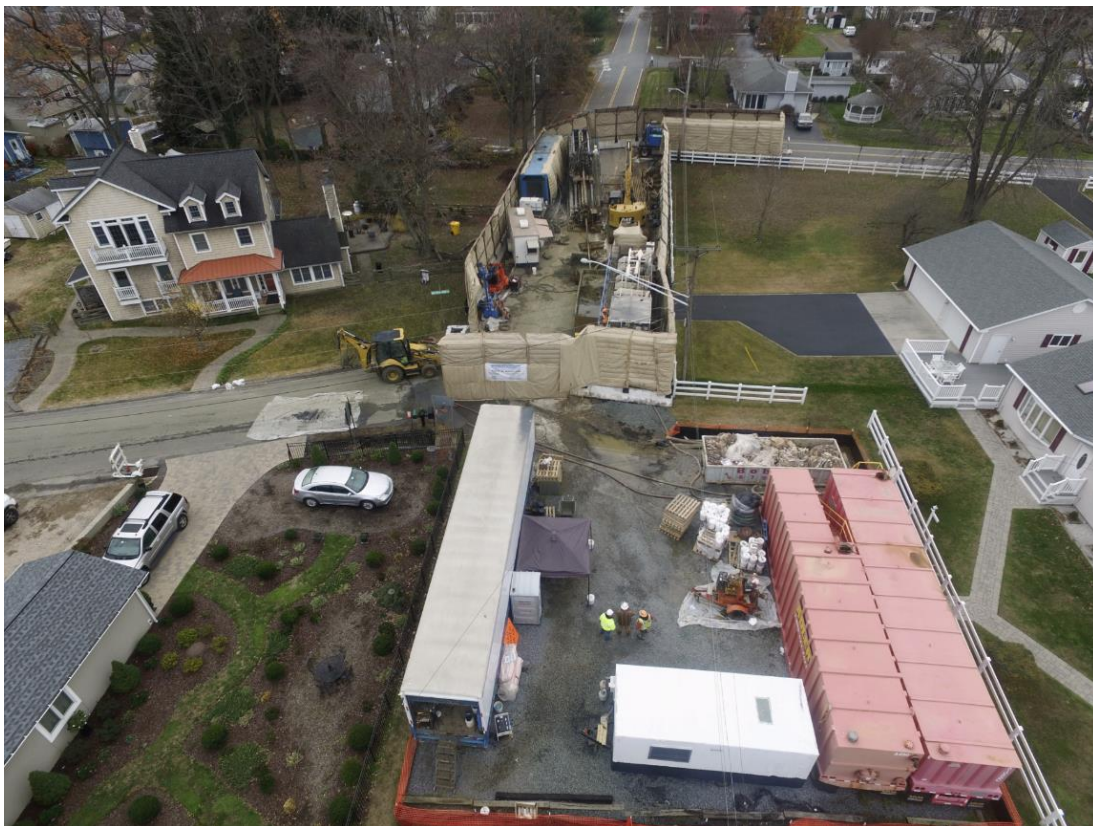
Figure 13. Examples of Large Land-based HDD Work Spaces. Note the tan inflated sound barriers in the lower image.
