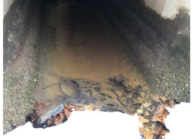
Film on water surface at 64 Gundalow – 1 culvert.
