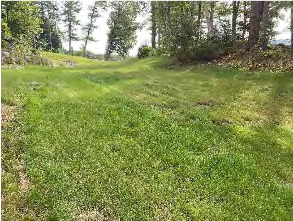
Fig 3: Slope below the manhole at Gundalow Landing/east side of the bay. Viewing east. (08-17-21)
