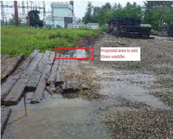
Fig 7: Proposed area in lay down yard to add straw bales/waddle, this would help filter The runoff water that channels under the timber matting. Viewing north. (6-11-19).
