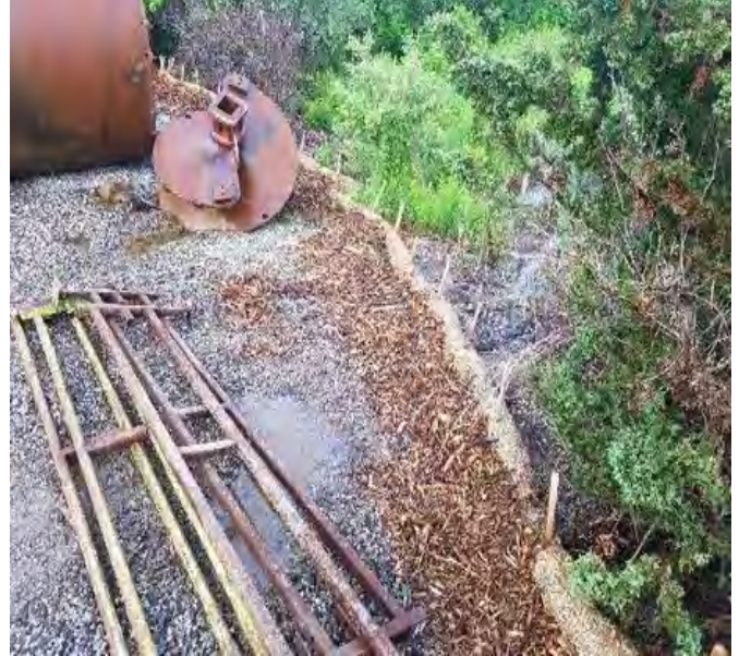
Fig 2: Combined berm installed around lay down area off of Gosling Rd. Viewing south. (6-14-19).
