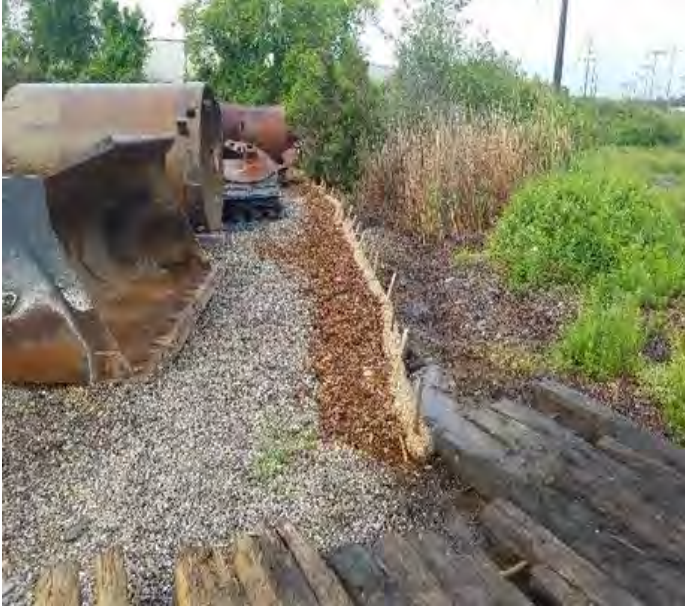
Fig 1: Combined berm installed around lay down area off of Gosling Rd. Viewing south. (6-14-19).
