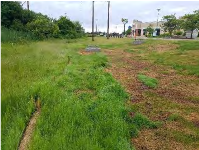
Fig 13: Str. F107-135 foundation and work site. Straw wattle are installed correctly and area has been seeded and broadcast with straw. Viewing southwest. (6-21-19).
