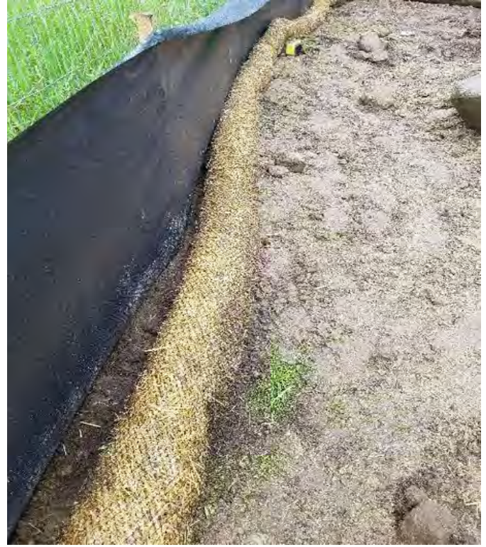
Fig 6: Silt fence and straw wattle installed between soil stockpiled in Waterworks Rd lay down area and wetland DW65. Viewing east. (6-21-19).
