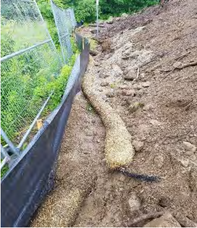
Fig 5: Silt fence and straw wattle installed between soil stockpiled in Waterworks Rd lay down area and wetland DW65. Viewing east. (6-21-19).
