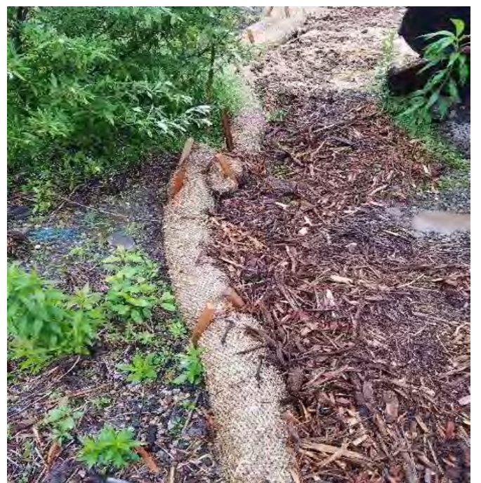
Fig 8: Combined berm installed correctly in lay down area off of Gosling Rd. Viewing north. (6-20-19).
