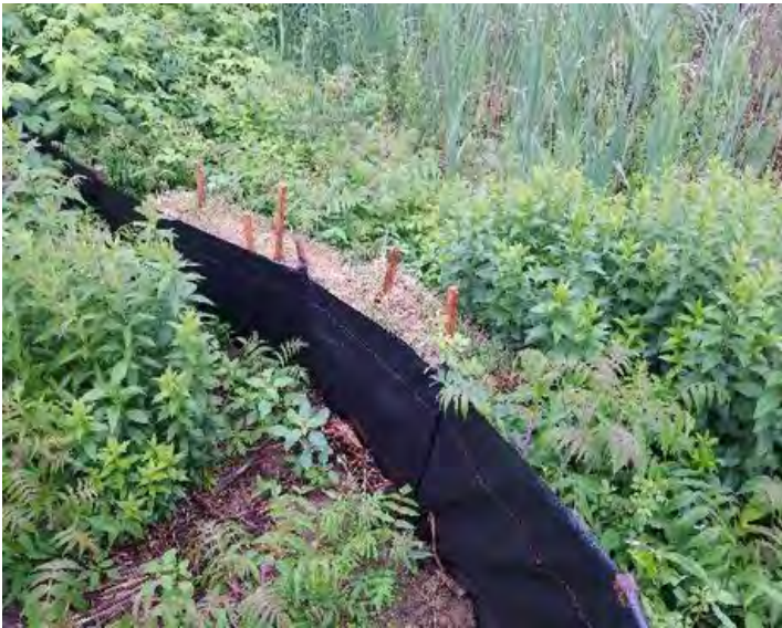
Fig 11: Silt fence and straw bales installed in low lying area between Str. F107-137 and wetland NW37. Viewing northeast. (6-21-19).
