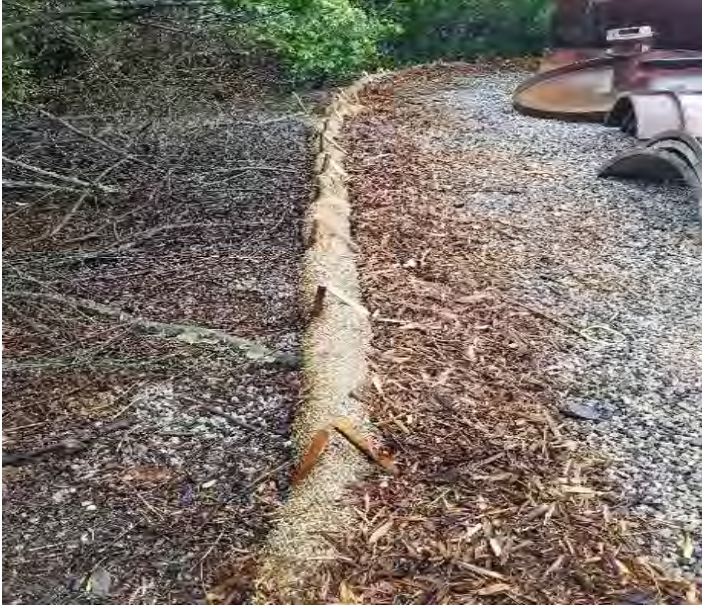
Fig 9: Combined berm installed correctly in lay down area off of Gosling Rd. Viewing east. (6-20-19).
