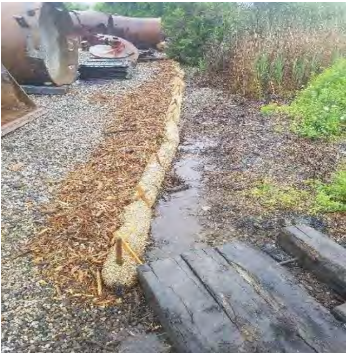
Fig 7: Combined berm installed correctly in lay down area off of Gosling Rd. Viewing south. (6-20-19).
