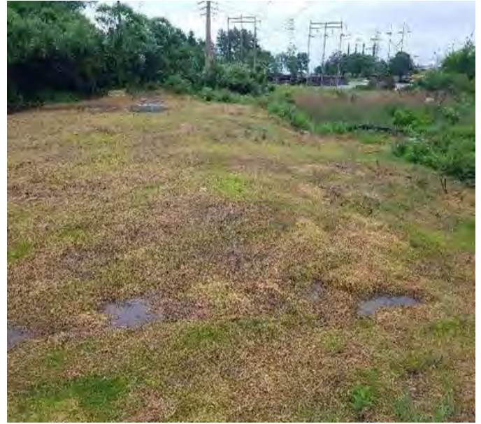
Fig 10: Str. F107-137 foundation and work pad seeded and broadcast with straw, grass beginning to grow. Viewing northeast. (6-20-19).
