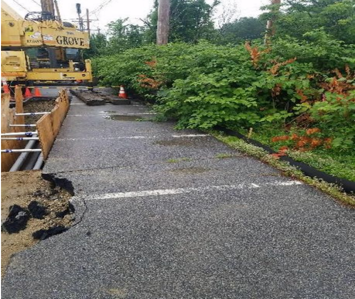
Fig 1: Filter sock installed next to drilling activities in "A" lot. Viewing north. (7-12-19).
