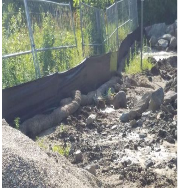
Fig 6: Silt fence installed on the north side of Waterworks Rd laydown area. (7-14-19).
