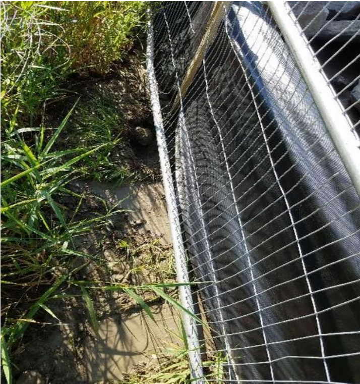
Fig 7: Area in silt fence installed in the Waterworks Rd laydown area that needs re-keyed into the ground. Viewing east. (7-14-19).
