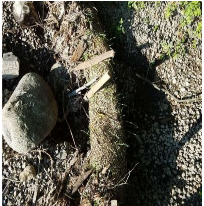
Fig 4: Portion of the combined berm that needs repaired in the laydown Area off of Gosling Rd. Viewing south. (7-14-19).
