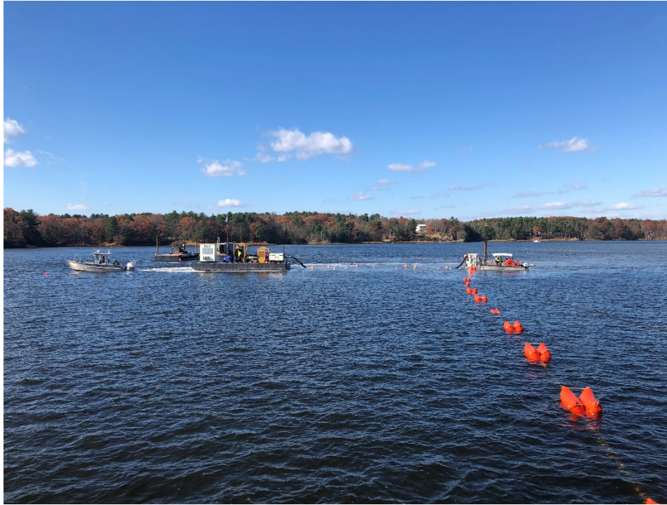
Cable 3 Installation. Cable with float bags tended to by divers and work boat removing bags prior to cable entering plow bell mouth. Pump barge tied to 2 nd work boat and moved with jet plow progress. Small spud barge with mini excavator in the background was used to tether to the cable for alignment purposes.
