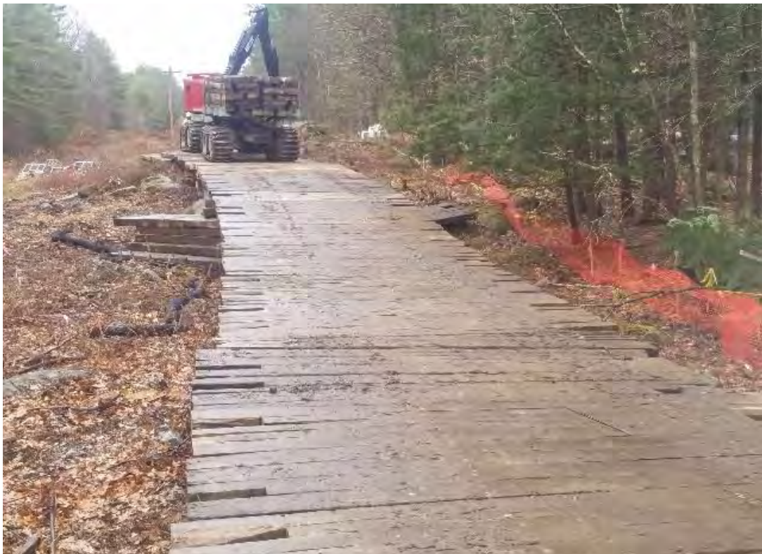
Fig 2: Installing timber mats on access road through wetland DW22, access to Strs. 89-90. Viewing east. (04-02-20).
