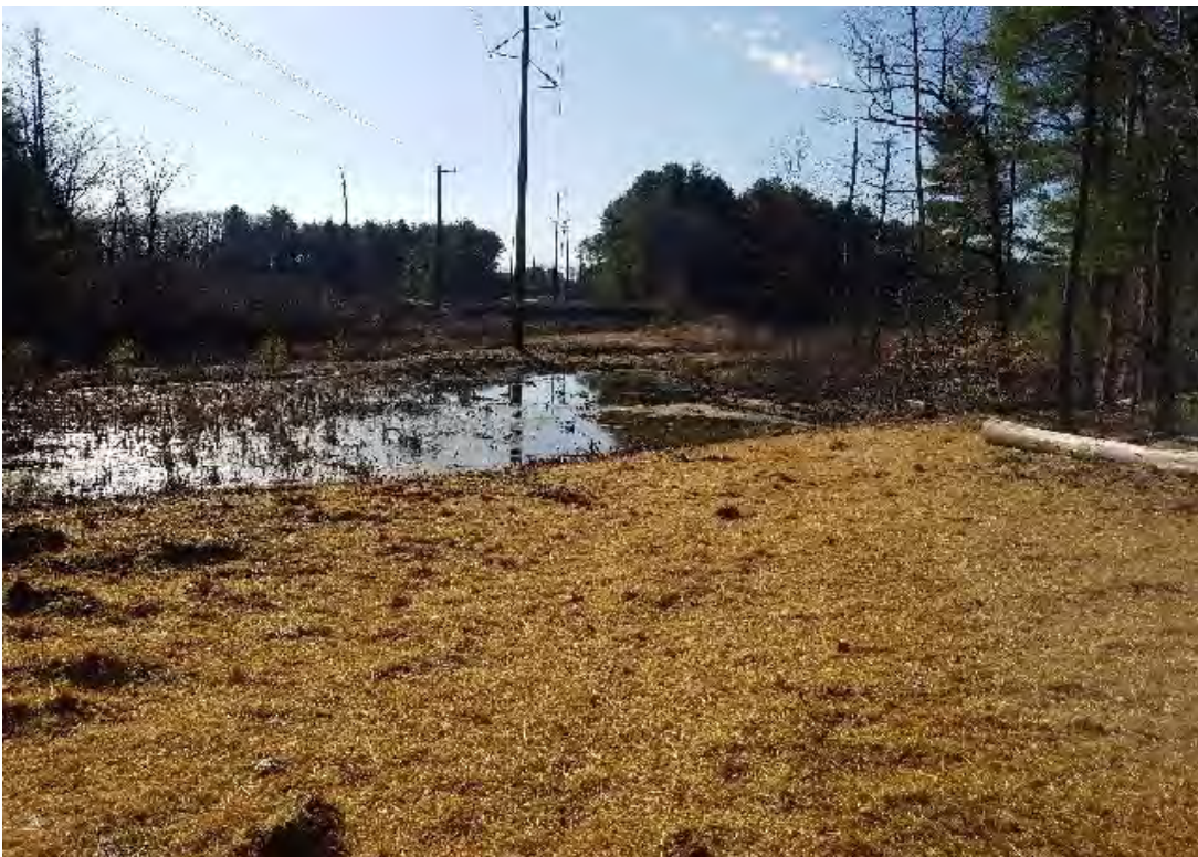
Fig 8: Timber mats removed and access road restored to Str. 114, through wetland NW17. Viewing southeast. (04-07-20).
