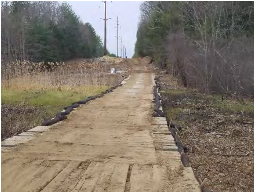
Fig 12: Access road through wetland DW21. Timber mats are being swept and maintained. Viewing west. (04-08-20).
