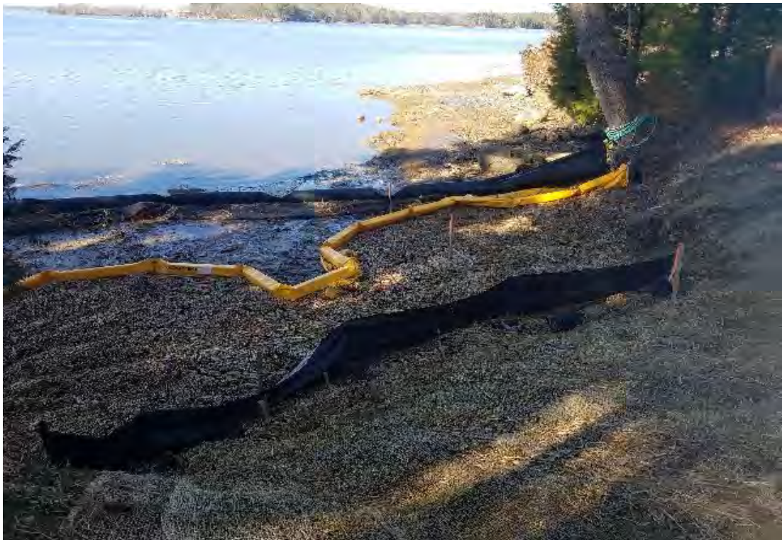
Fig 4: Turbidity barrier in intertidal zone at Gundalow landing/east side of the Bay. Viewing west. (04-06-20).
