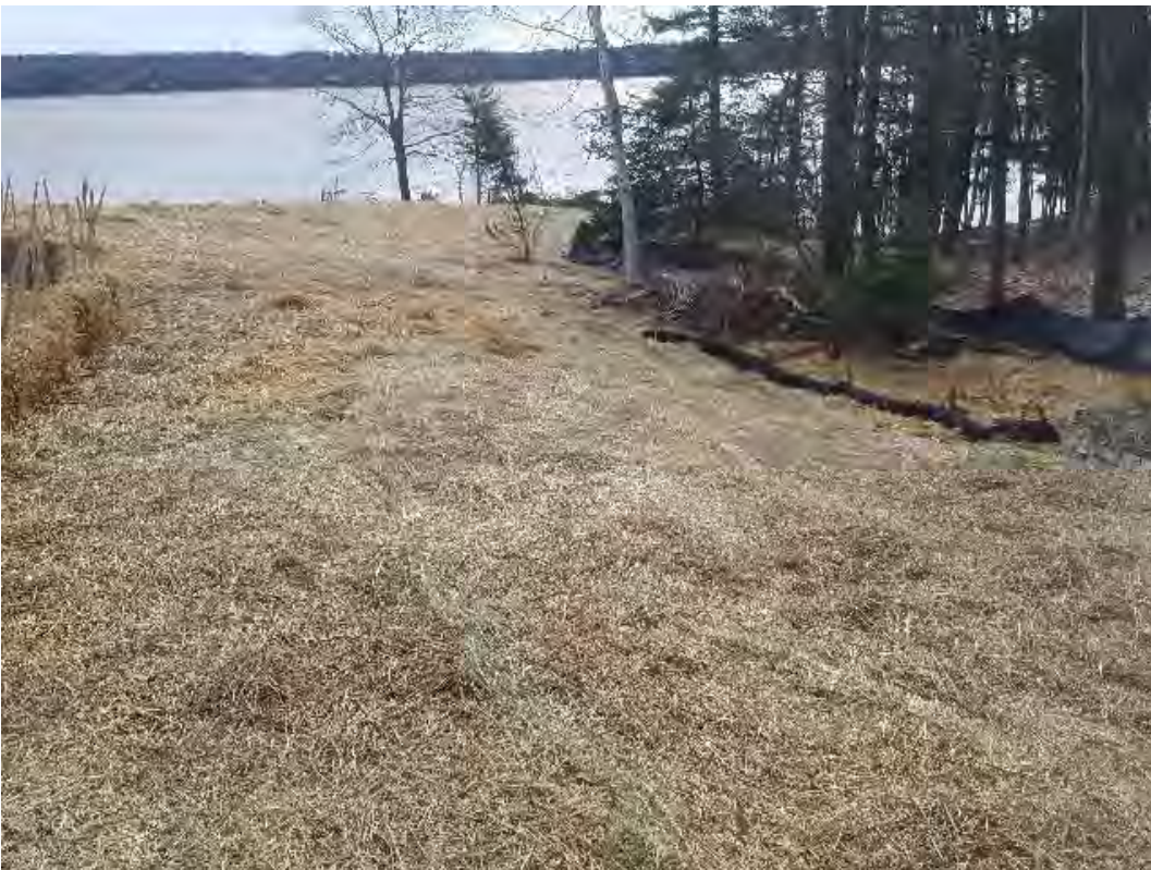
Fig 6: Previous erosion repairs are holding up on the slope at the Getchell property/west side of the Bay. Viewing east. (04-10-20).
