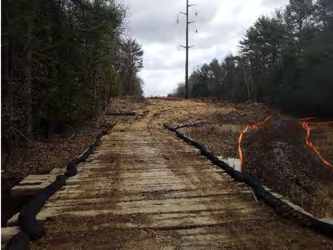
Fig 9: Access road over stonewall WP-28 and through wetland DW25 to Str. 76. Viewing east. (04-10-20).
