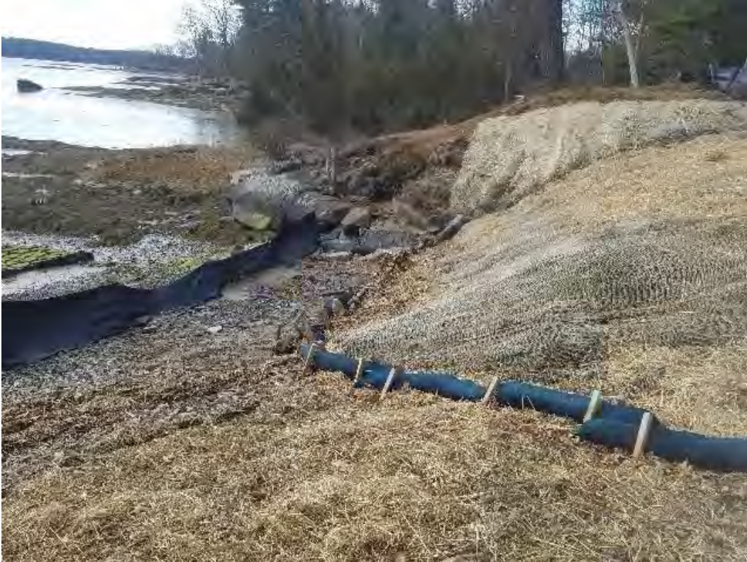
Fig 7: BMPs at toe of slope at Getchell property/west side of the Bay. Viewing south. (04-10-20).
