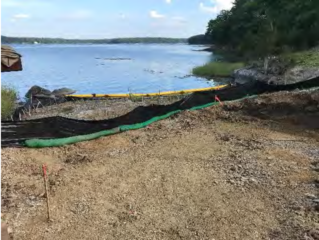
Fig 5: Installation of silt fence and sock along at downstream edge of cable house foundation excavation to protect the salt marsh. Viewing southeast. (08-10-20).
