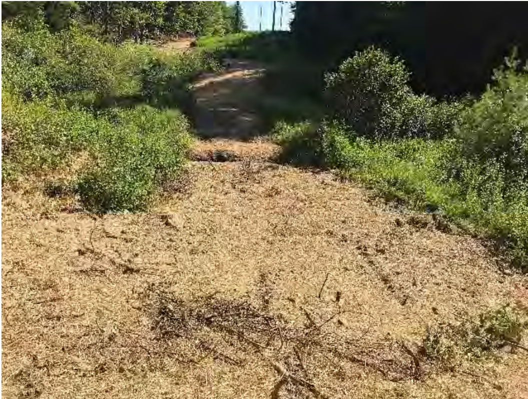
Fig 1: Access road across stream DS46 near Str. 51 seeded and mulched. Viewing northeast. (08-06-20).
