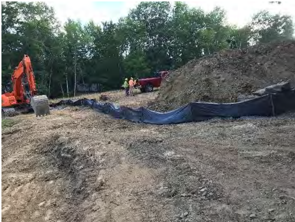
Fig 6: Installation of silt fence around base of soil excavated for cable house foundation at Eversource property/west side of the bay. Viewing southwest. (08-10-20).
