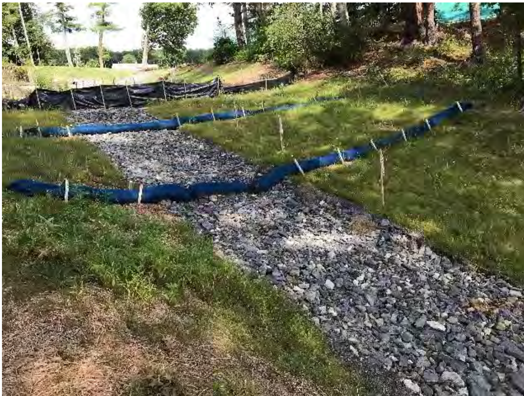
Fig 8: Slope below manhole at Gundalow Landing/east side of the bay. Viewing east. (08-12-20).
