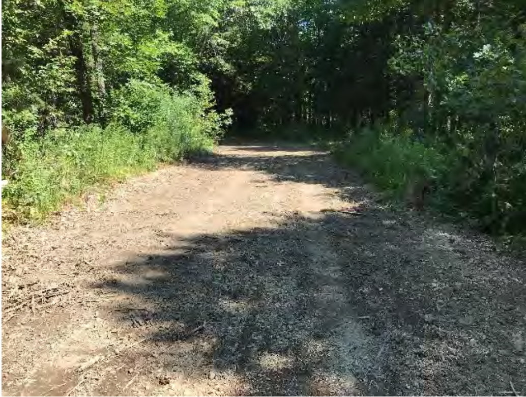
Fig 3: Timber mat removal along Bennett Rd. access road up to staging area. Viewing north. (08-10-20).
