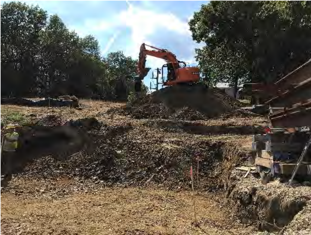
Fig 4: Excavation for the new cable house foundation at the Eversource property/west side of the bay. View west. (08-10-20).
