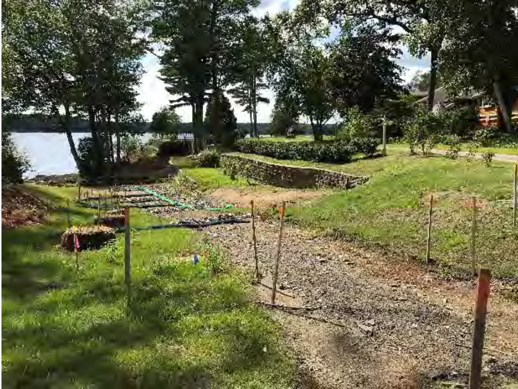
Fig 7: Slope above the manhole at Gundalow Landing/east side of the bay. Viewing west. (08-12-20).
