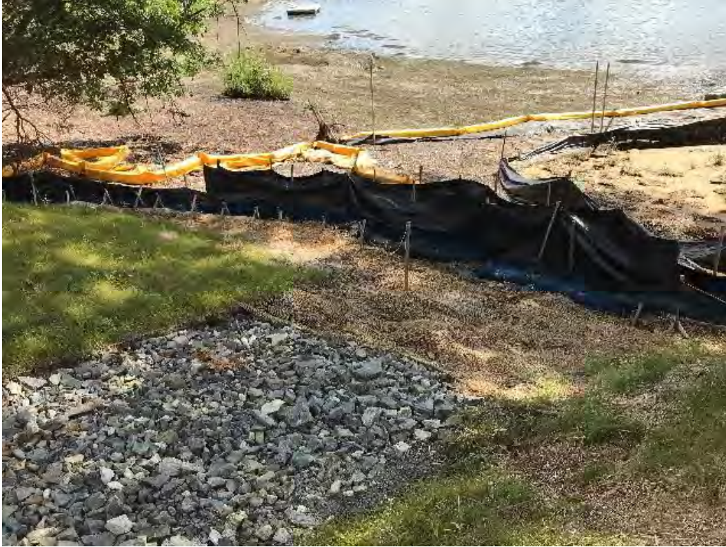
Fig 9: Toe of slope below manhole at Gundalow Landing/east side of the bay. Viewing south. (08-12-20).
