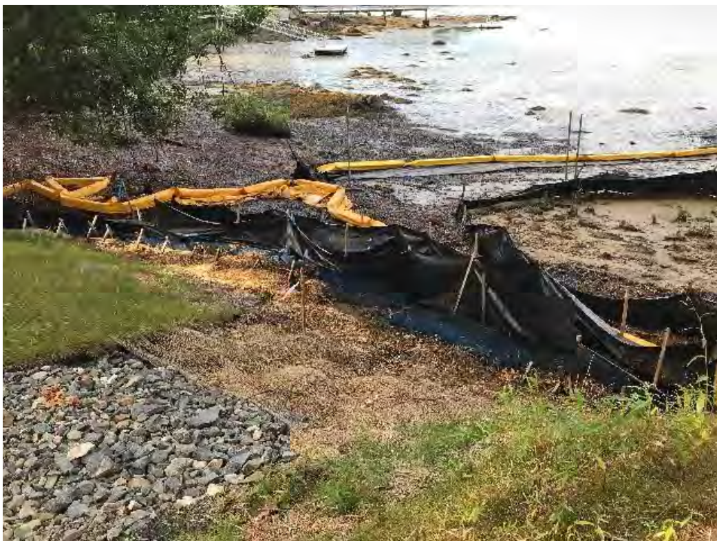
Fig 6: Toe of slope below manhole at Gundalow Landing/east side of the bay. Viewing south. (08-19-20).
