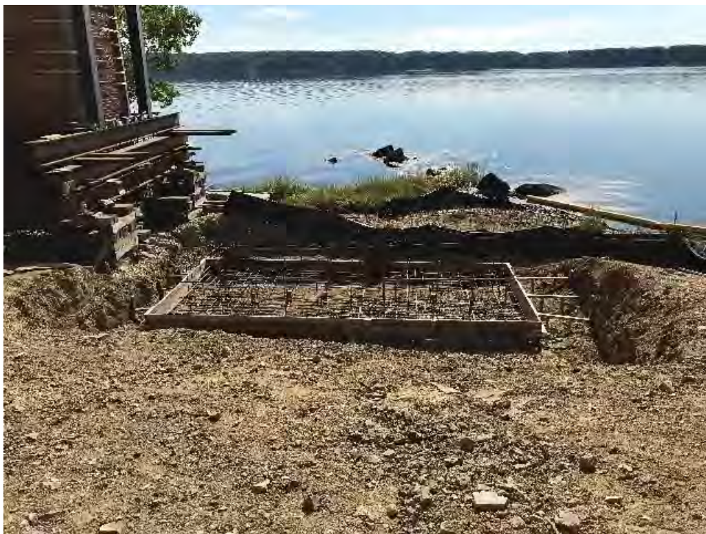
Fig 10: Form for the first part of the new cable house foundation at Eversource property/west side of the bay. Viewing east. (08-13-20).
