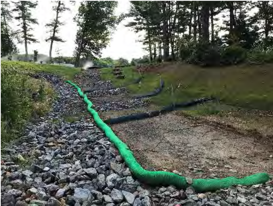
Fig 5: Slope above the manhole at Gundalow Landing/east side of the bay. Viewing east. (08-19-20).
