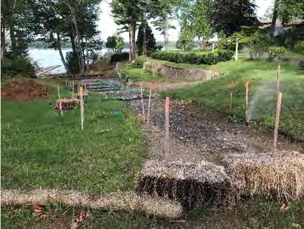
Fig 3: Slope above the manhole at Gundalow Landing/east side of the bay. Viewing west. (08-19-20).
