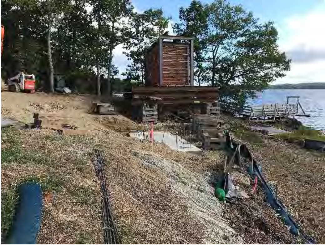
Fig 11: Site of the new cable house location at Eversource property/west side of the bay and the new cable house foundation partially constructed. Viewing north. (08-17-20).
