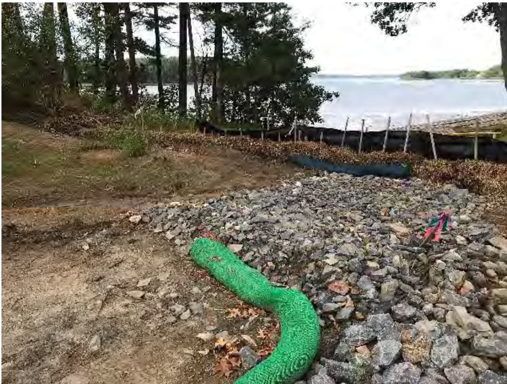
Fig 4: Toe of slope above the manhole at Gundalow Landing/east side of the bay. Viewing south. (08-19-20).
