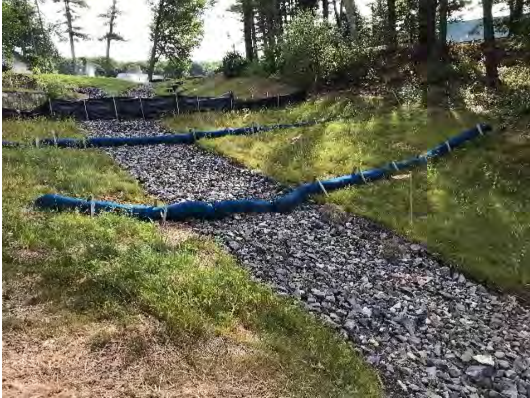
Fig 7: Slope below manhole at Gundalow Landing/east side of the bay. Viewing east. (08-19-20).
