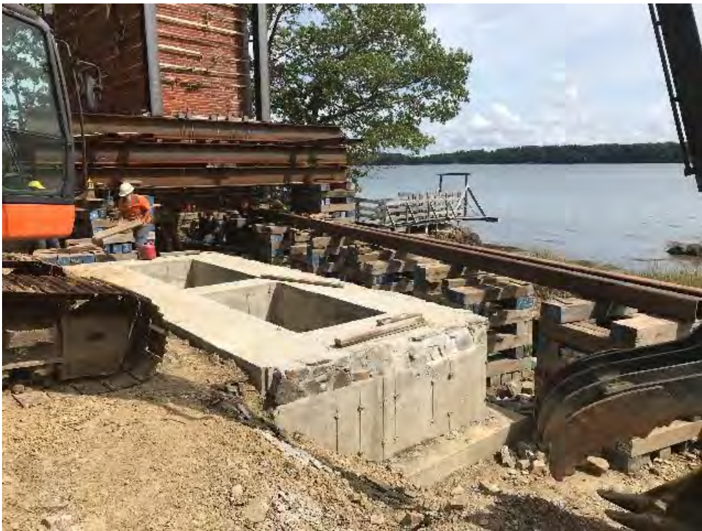
Fig 2: Continued preparation of the system to move the cable house to its new location at the Eversource property/west side of the bay. Viewing northeast. (09-01-20).
