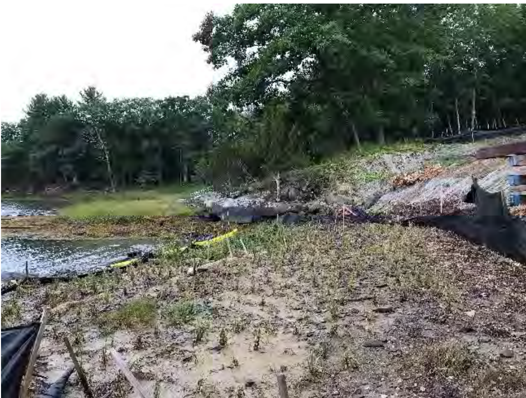
Fig 8: Salt marsh restoration at Eversource property/west side of the bay. Viewing south. (09-02-20).
