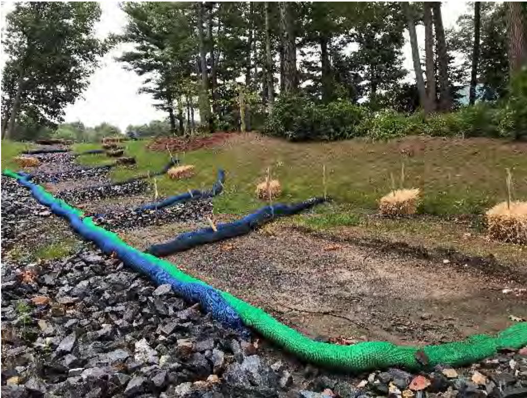
Fig 4: Slope above the manhole at Gundalow Landing/east side of the bay. Viewing east. (09-02-20).
