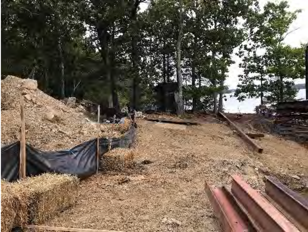
Fig 9: Silt fence stabilizing the soil stockpile at the Eversource property/west side of the bay is functioning. (09-02-20).
