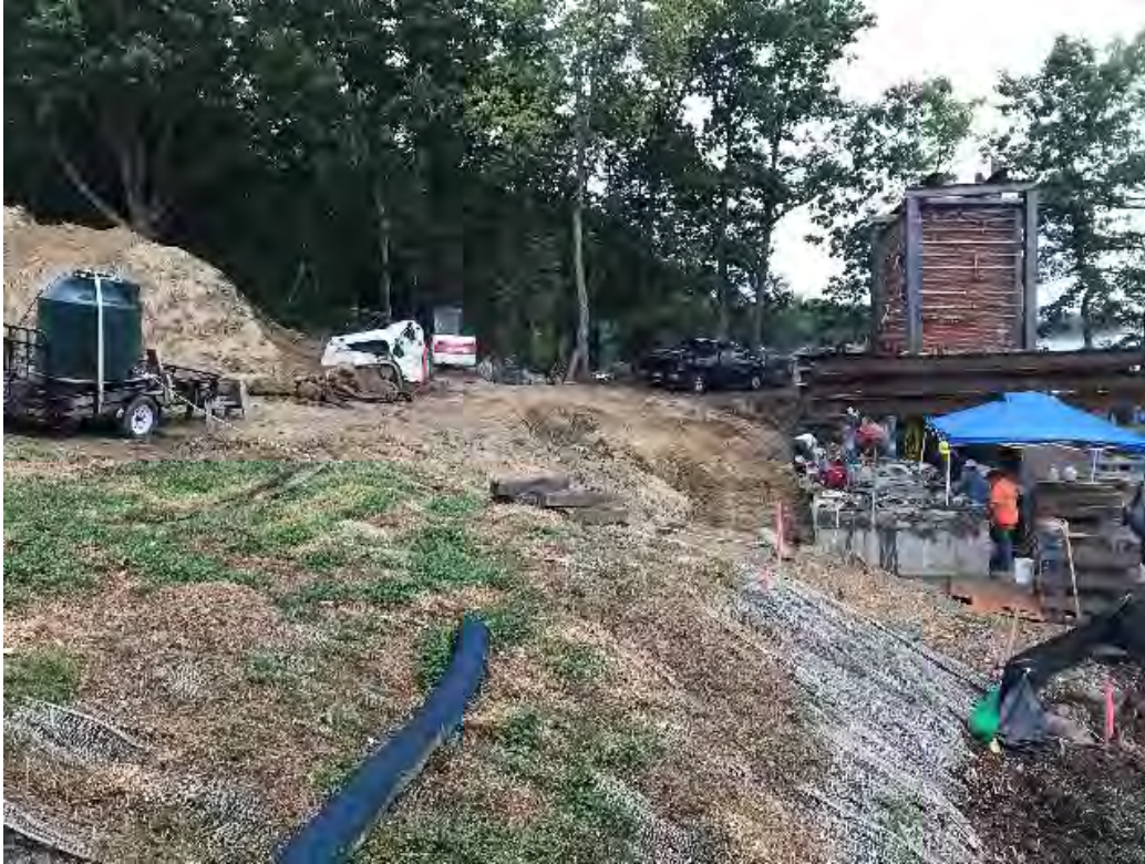
Fig 1: Installation of a stone façade on the new cable house foundation and backfilling along its western side at the Eversource property/west side of the bay. Viewing north. (08-27-20).
