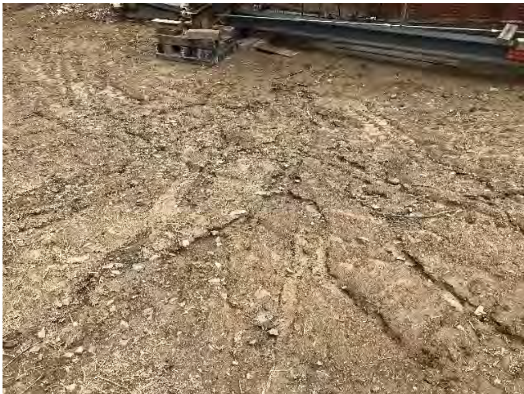
Fig 6: Rills observed upslope of the cable house foundation at the Eversource property/west side of the bay. Viewing east. (09-11-20)
