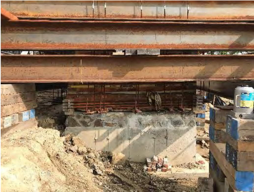
Fig 7: Cable house positioned over the foundation at the Eversource property/west side of the bay. Viewing north. (09-14-20)
