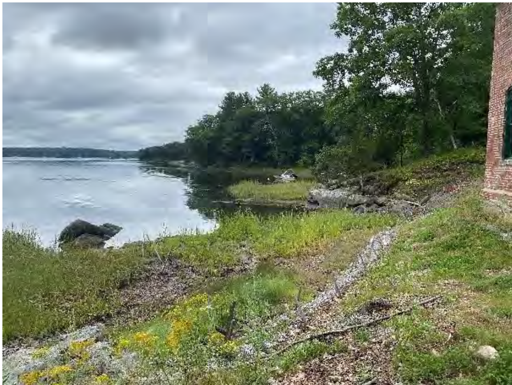
Fig 4: Toe of the slope and salt marsh restoration at the west side of the bay. Viewing south. (08-20-21)
