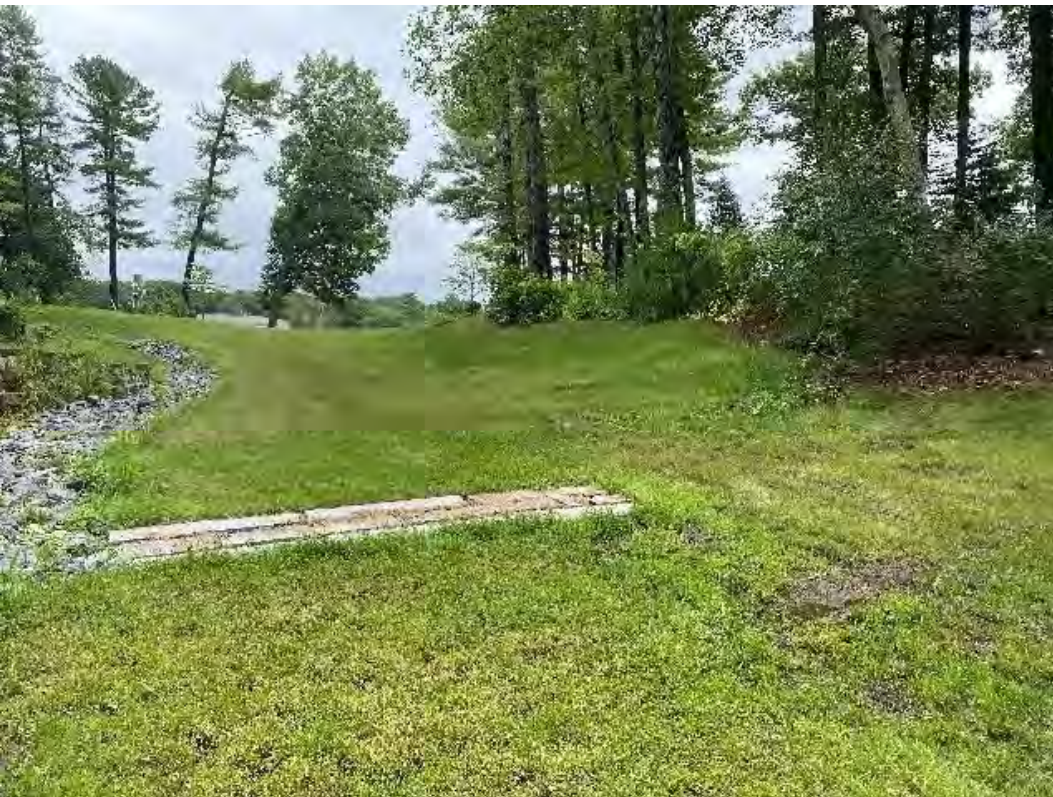
Fig 8: Slope below the manhole at Gundalow Landing/east side of the bay. Viewing east. (08-20-21)
