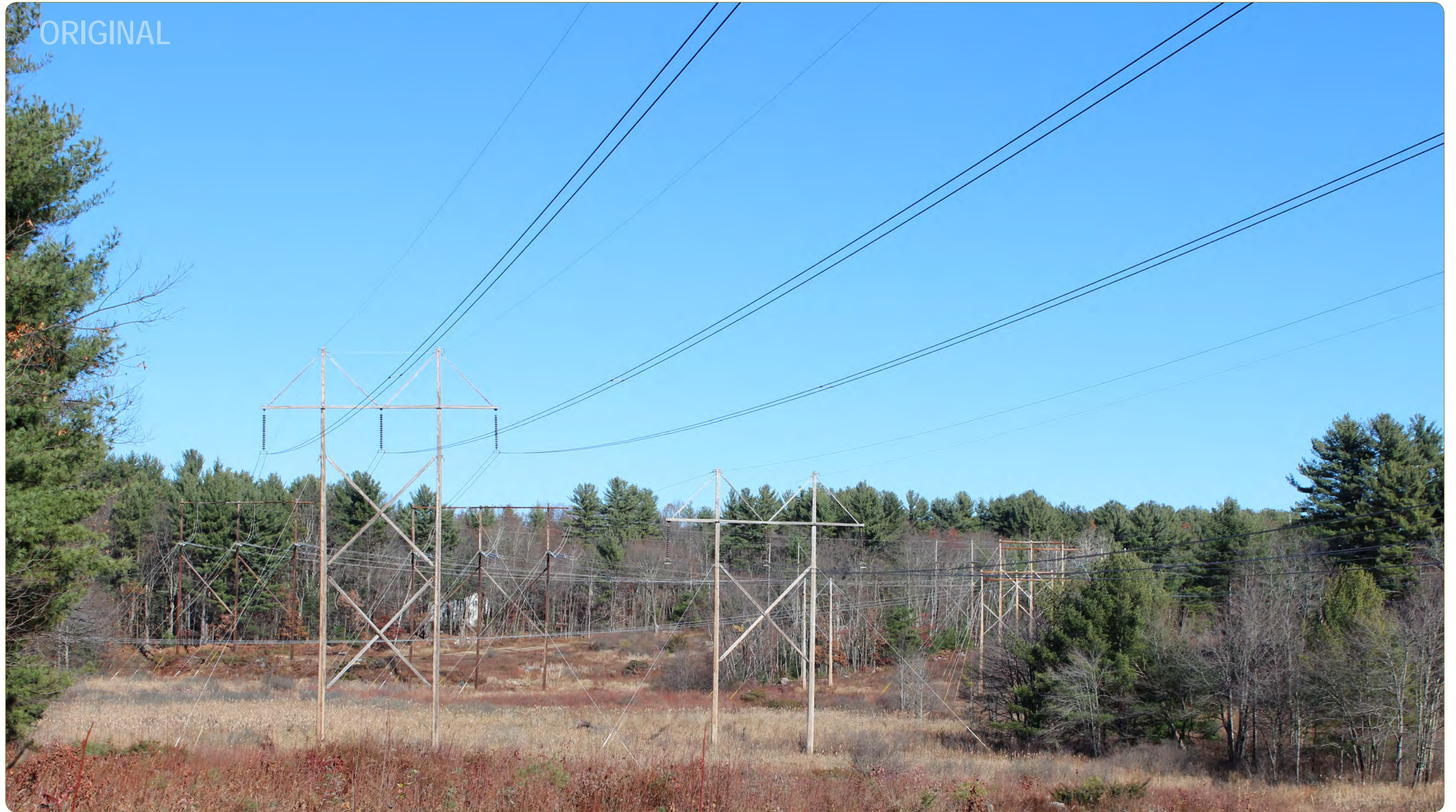
Merrimack Valley Reliability Project Towns of Pelham, Windham, Hudson and Londonderry, New Hampshire Figure 15: Viewpoint 109 (Musquash Conservation Area, Town of Londonderry - View to the northeast) May 2015
