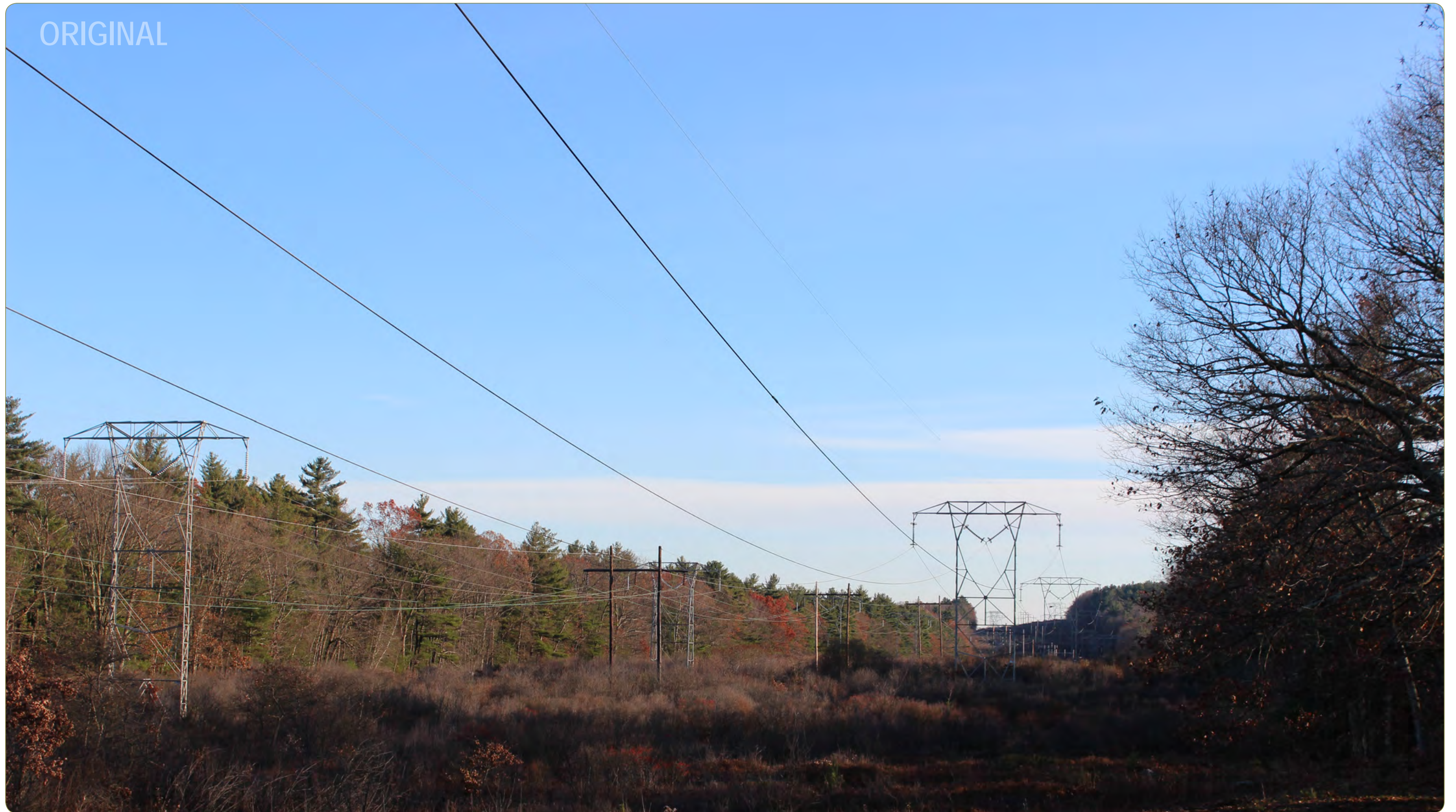
Merrimack Valley Reliability Project Towns of Pelham, Windham, Hudson and Londonderry, New Hampshire Figure 9: Viewpoint 5 (Arthur Peabody Town Forest, Town of Pelham - View to the southeast) May 2015
