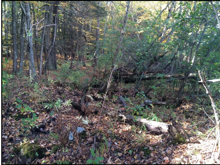
Photo 9: View northwest toward WA 36A. Construction work pad for pole installation in wetland to extend into this section of the wetland. Tree clearing proposed in wetland along ROW. 10/08/2014.
