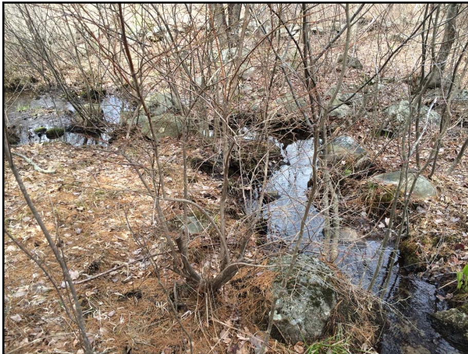
Photo 26: View north of intermittent stream SA-39. Construction work pad for pole installation to extend across stream. Timber access matting planned where ROW access road crosses stream. 04/22/2015.
