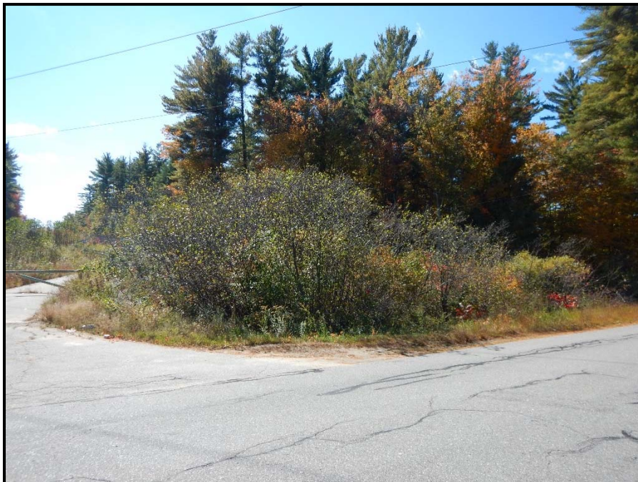
Photo 48: View southwest toward WA 69A. Construction work pad for pole installation outside of wetland to extend into a section of this wetland. Timber access matting planned along access road adjacent to WA 69. 10/09/2014.
