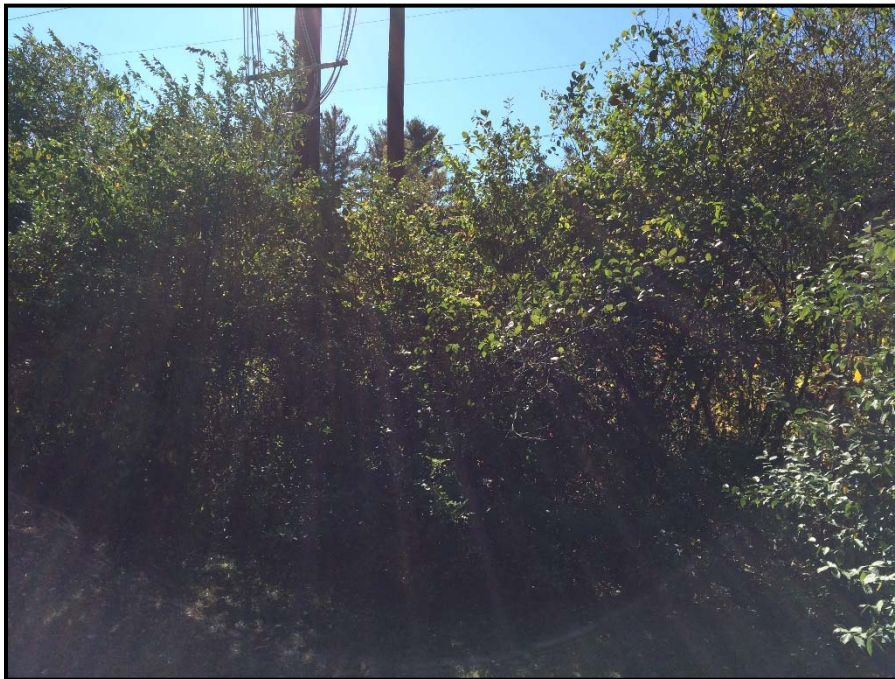
Photo 40: View west toward WA 59D. Construction work pad for pole installation planned in this section of the wetland. 10/09/2014.
