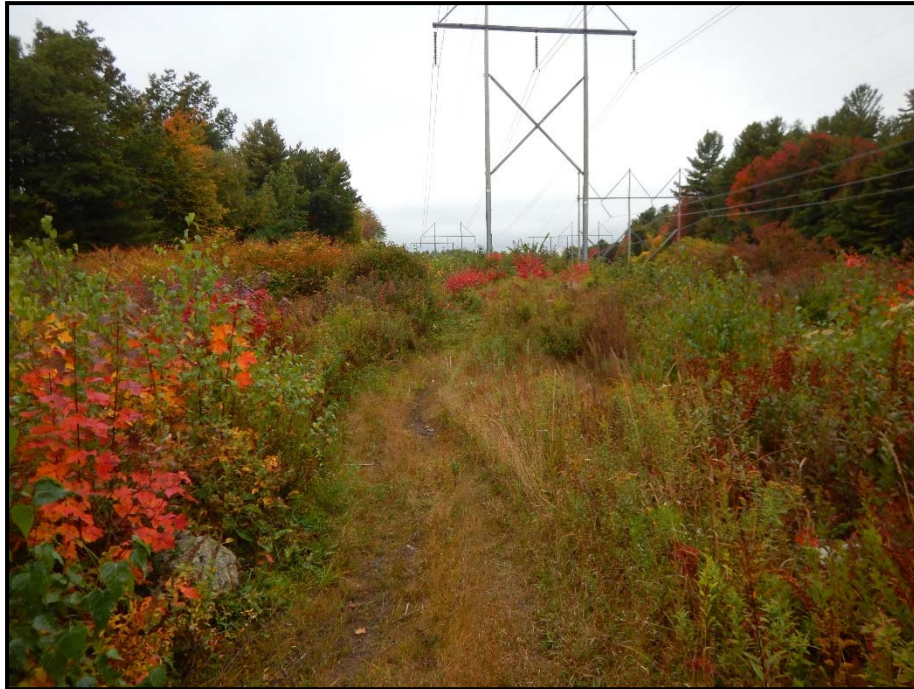
Photo 109: View west along Eversource access road through WA 132 where timber access matting is planned. Tree clearing also planned within this wetland. 09/30/2014.
