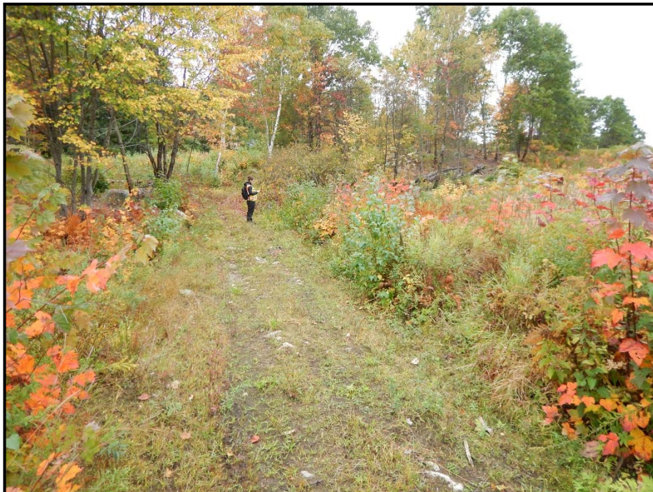
Photo 92: View south of Eversource access road through WA 114 where timber access matting is planned. Narrow strip of trees visible is proposed to be cleared. 10/01/2014.
