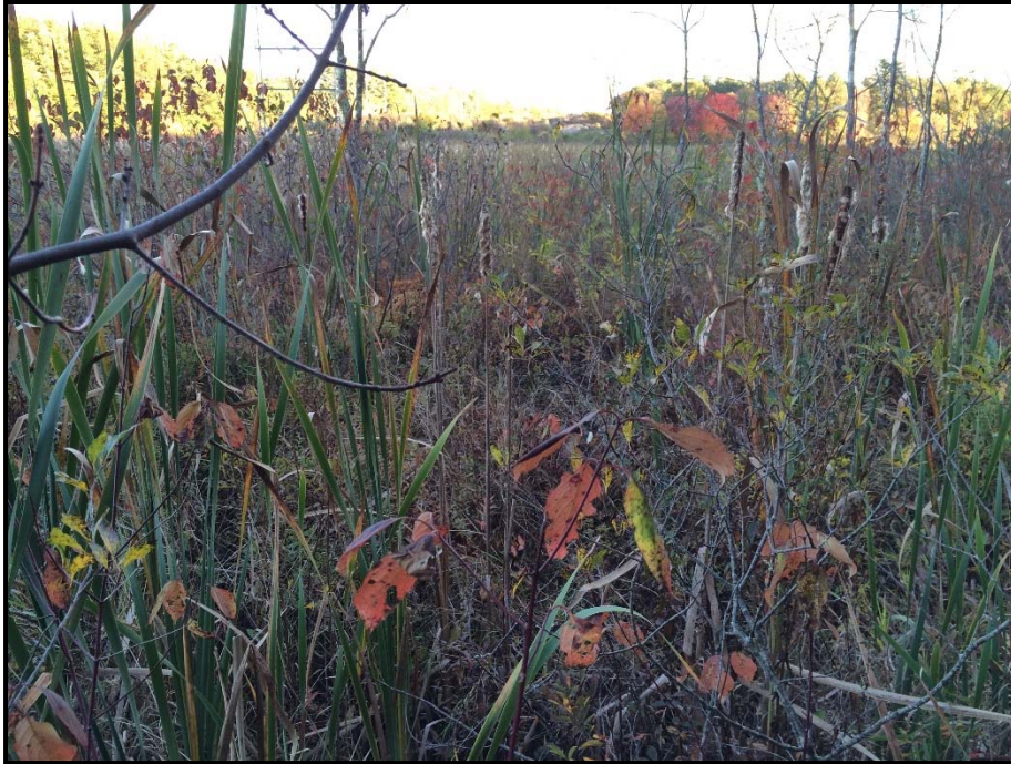
Photo 21: View south toward WA 46. Construction work pad for pole installation in upland to extend into this section of the wetland. Timber access matting is planned along access road through eastern section of wetland. Tree clearing proposed in wetland along ROW. 10/08/2014.
