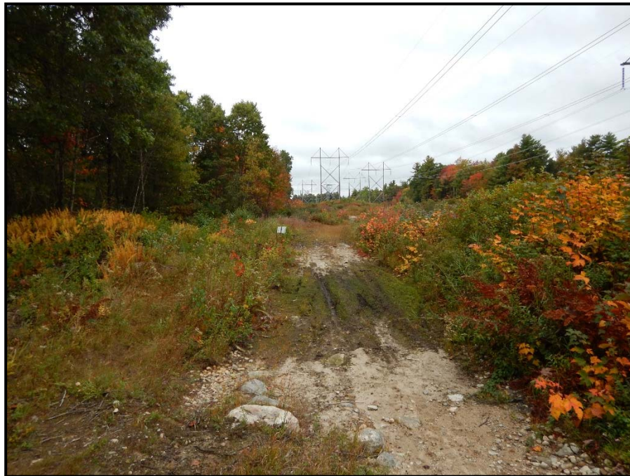
Photo 90: View south of Eversource access road through second section of WA 111 where timber access matting is planned. Further south a construction work pad is planned for pole installation. 10/02/2014.
