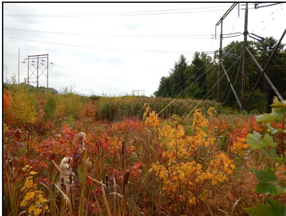
Photo 134: View south toward WA 167 near the Scobie Pond Substation. A construction work pad is to be placed over part of this wetland for a pull pad site. 09/24/2014.
