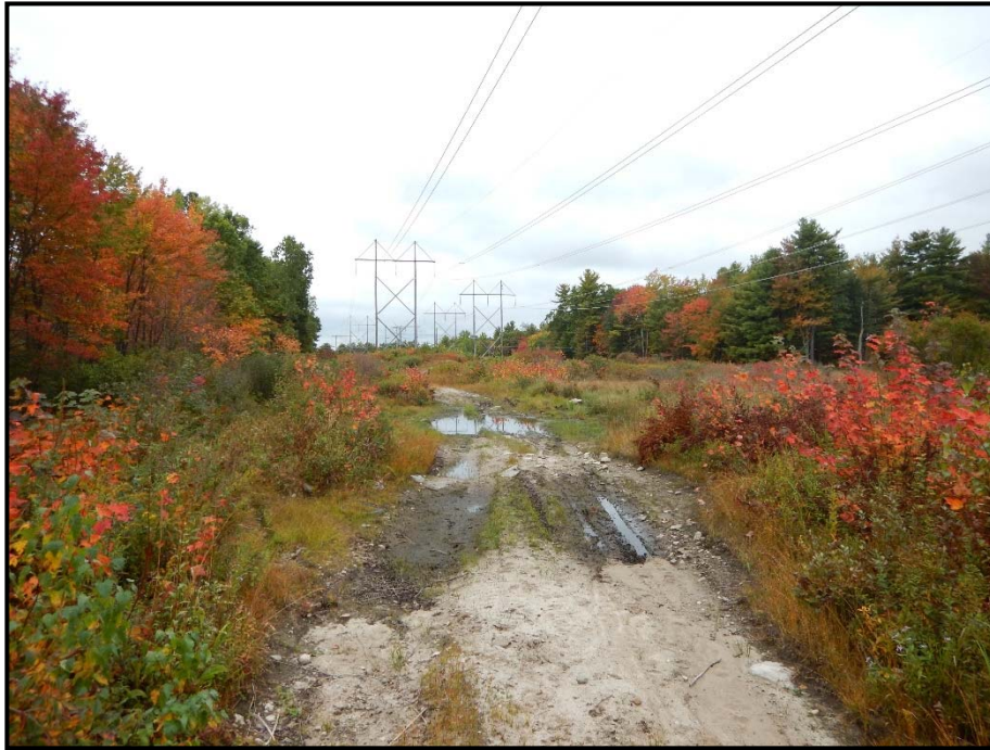
Photo 89: View south of the Eversource access road through first section of WA 111 where timber access matting is planned. Construction work pad site and proposed tree clearing left of photo. 10/02/2014.
