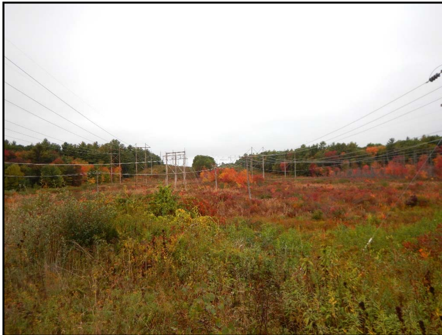
Photo 116: View west of WA 144. Location of construction work pad to install Structure 263. Access road nearby. East of photo is location of proposed construction work pad for pull pad site. 09/29/2014.
