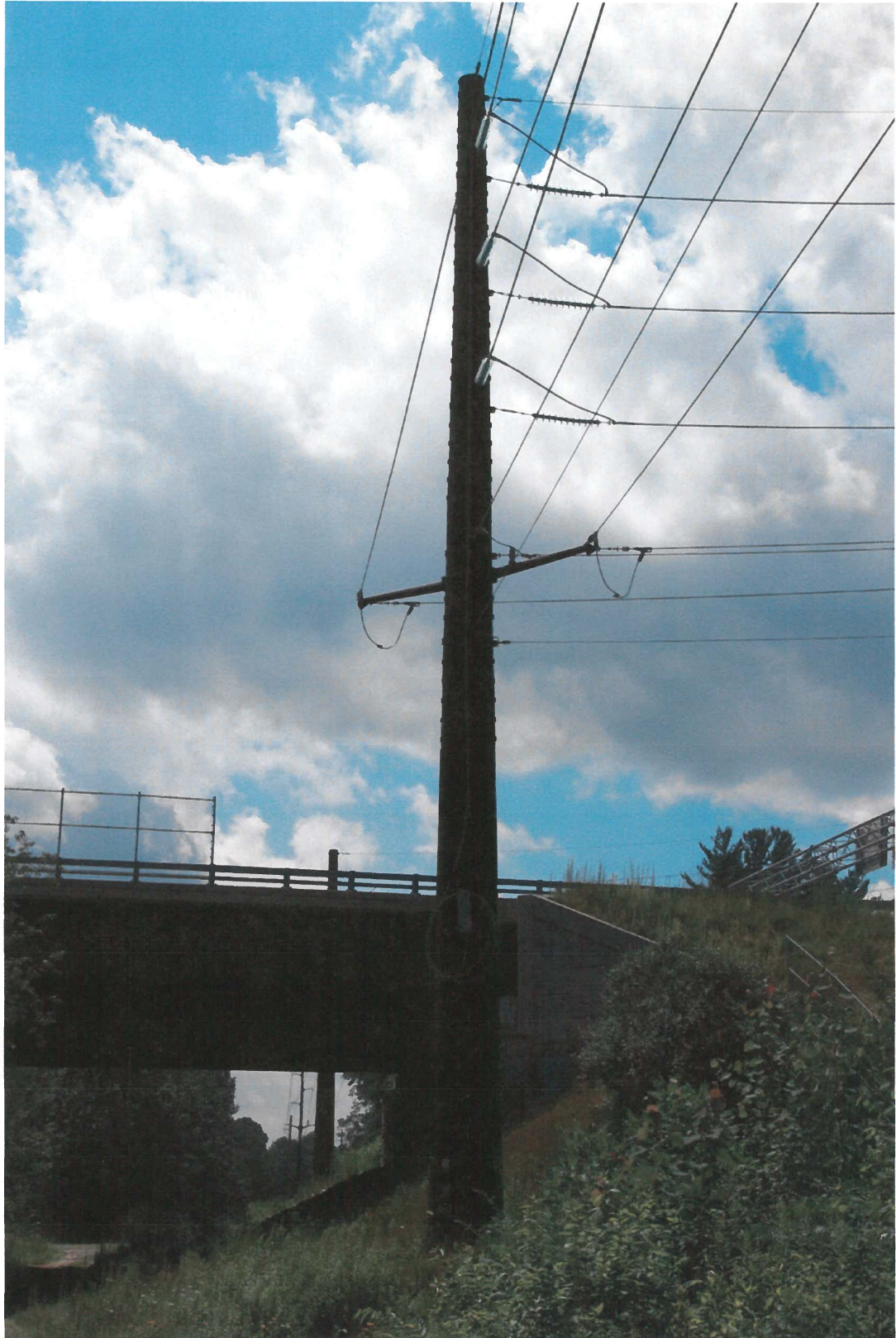
POWERLINE POLE IN BEDFORD NEAR AIRPORT ACCESS ROAD – APPROXIMATELY 70 FEET TALL THE POLE IS 5 TO 6 FEET WIDE AT THE BASE
