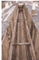
Buried 4 to 15 feet below
