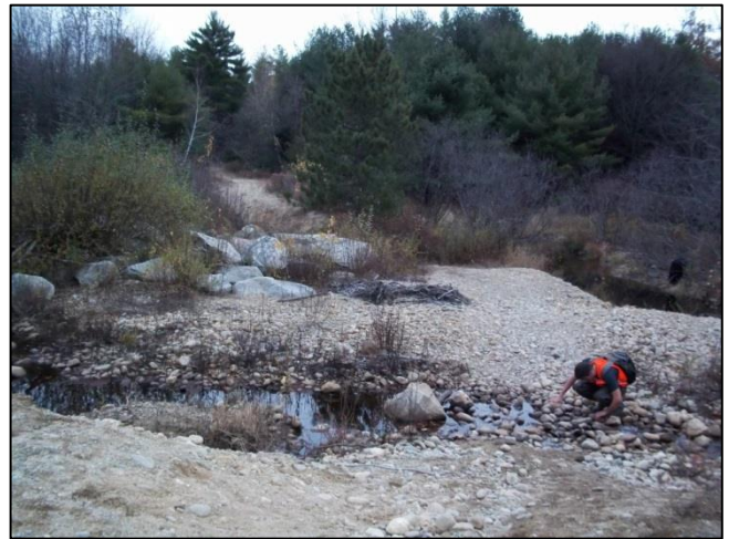
Photo point 33. A washed-out dirt road crossing through the Birch Brook wetland complex.
